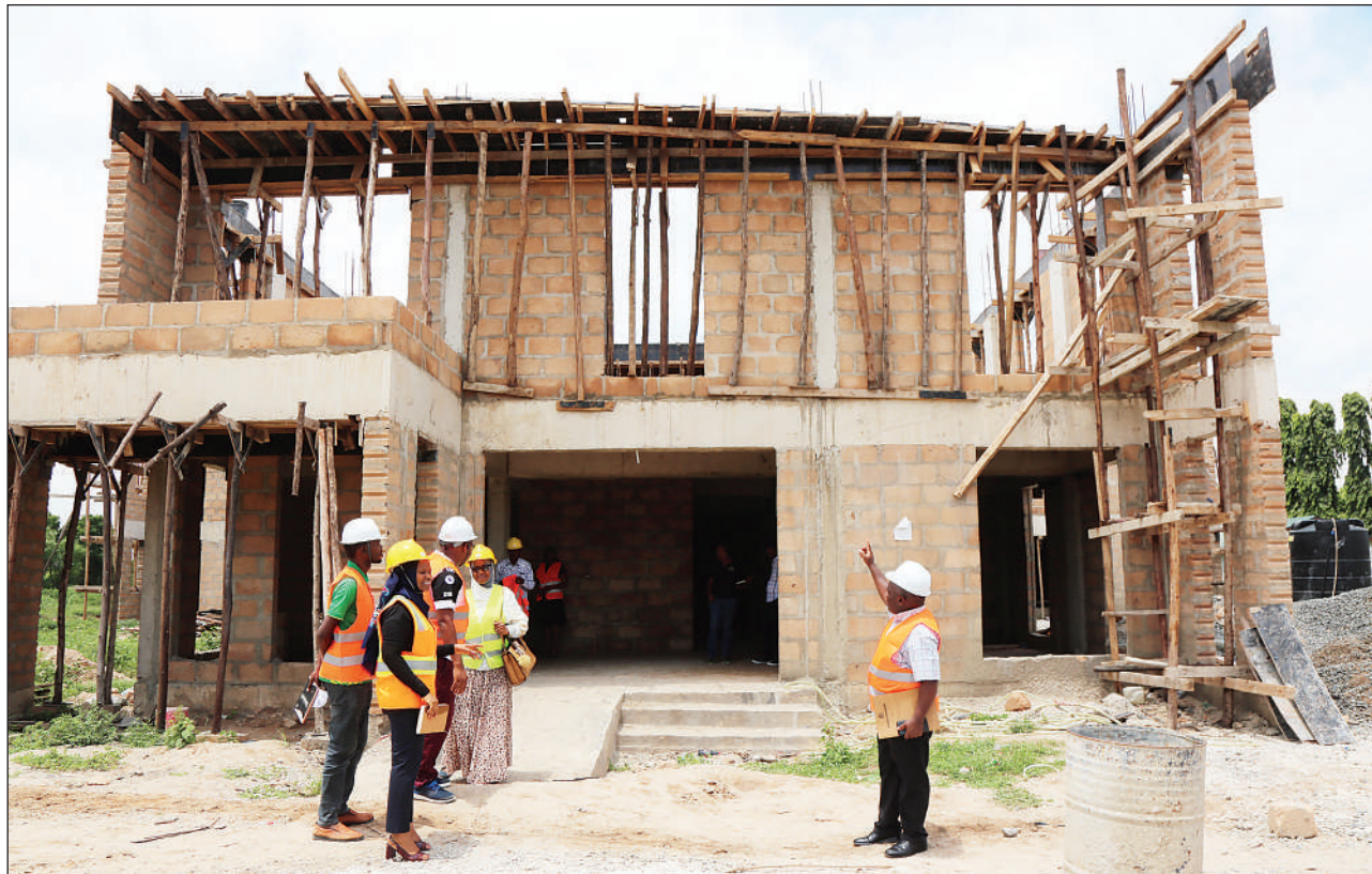
TFRA construction site of the International Fertilizer Laboratory in Agriculture III in Dar es Salaam
