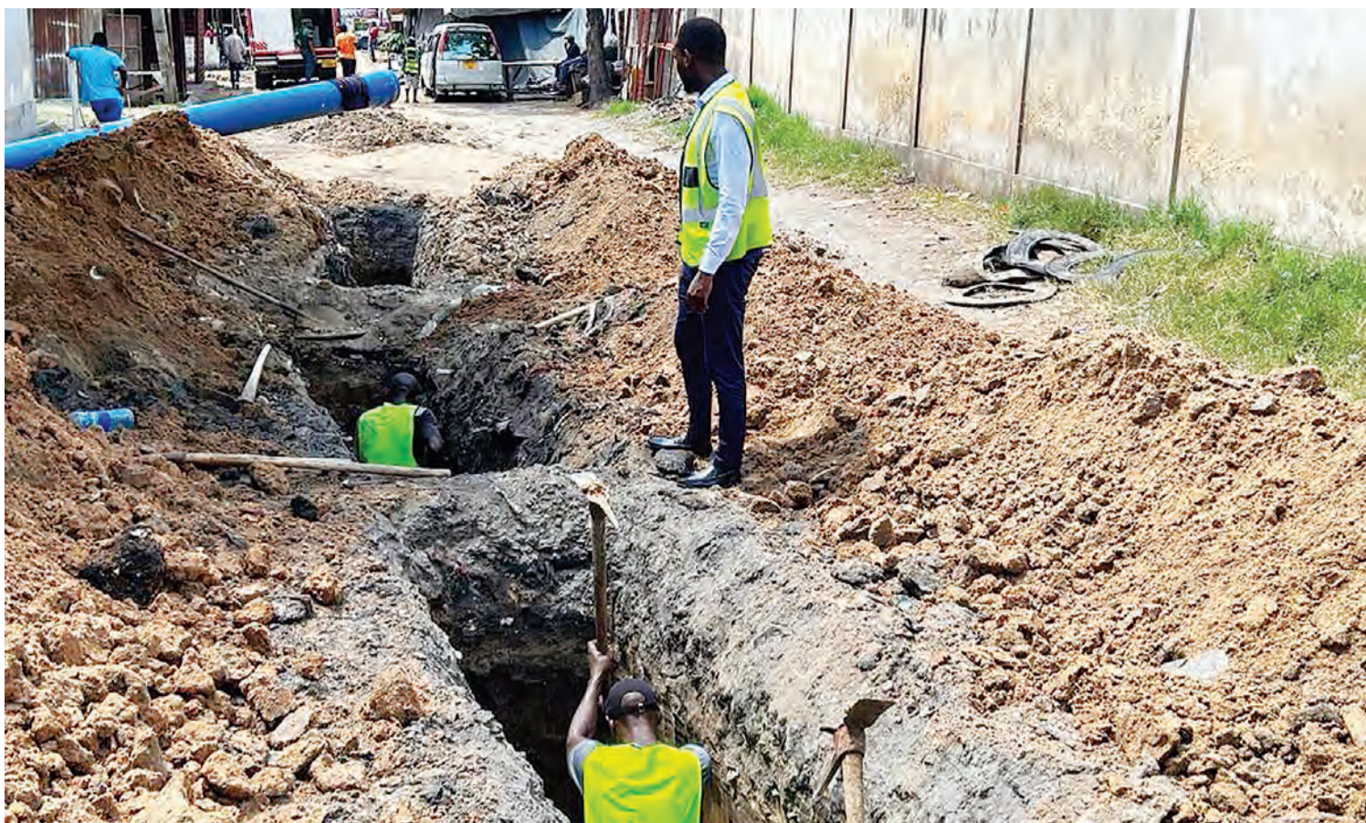
Implementation by the Dar es Salaam Water and Sanitation Authority (Dawasa) of the city's 'PSSSF Sinza-Kijitonyama' sanitation project is well under way, as captured yesterday. It is chiefly meant to curb environmental pollution and benefit 1,000 people when completed next month. Photo Correspondent Joseph Mwendapole
