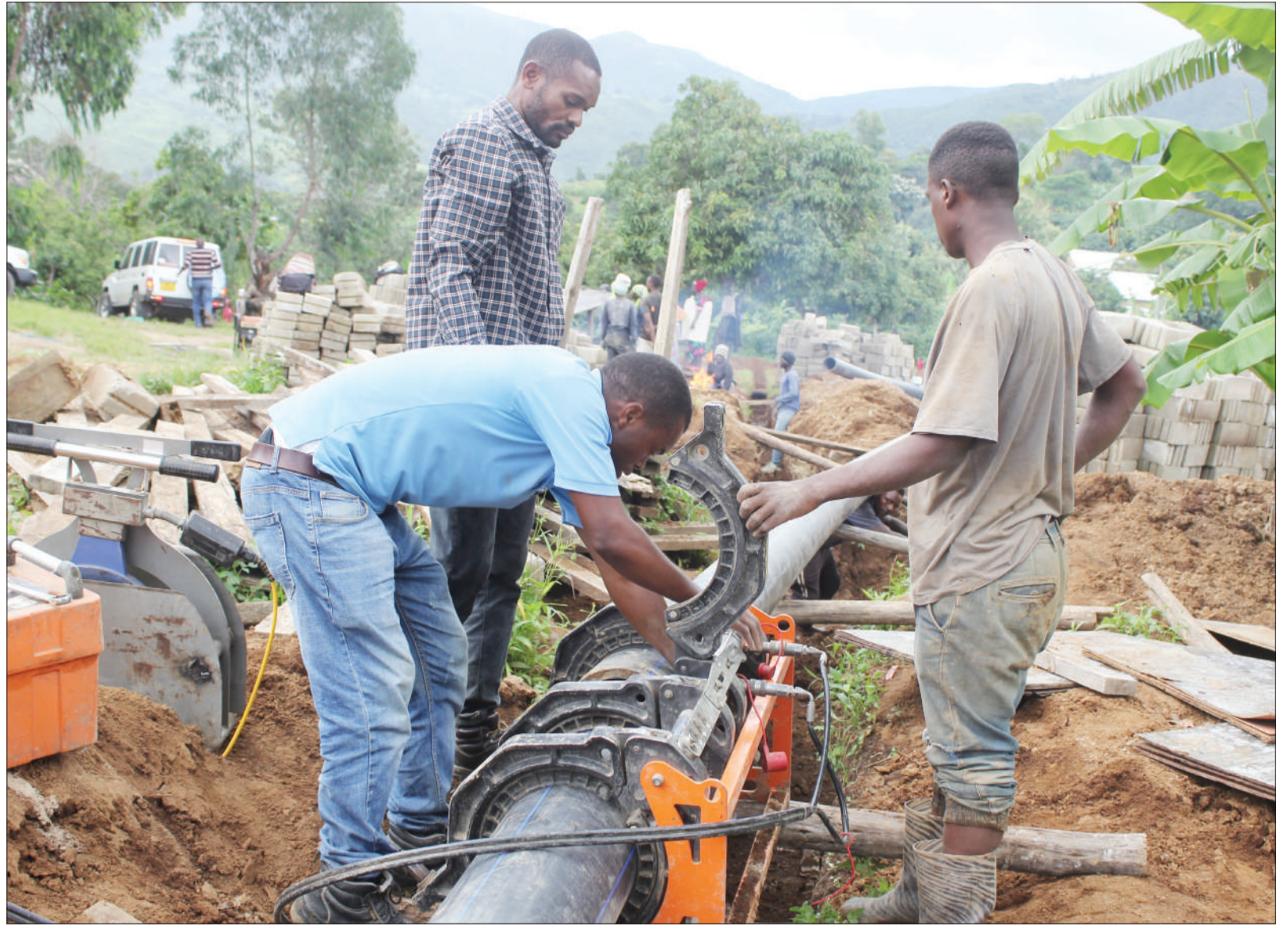
Technicians pictured at Mbalizi township in Mbeya Urban District yesterday working on an Ilunga water project pipe meant supply the precious liquid to various parts of the district. Photo: Correspondent Nebart Msokwa
