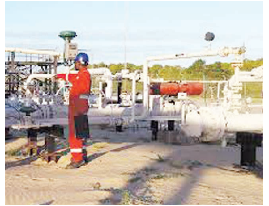
A technician with Maurel & Prom attending to gas infrastructure at Mnazi Bay in Mtwara.
