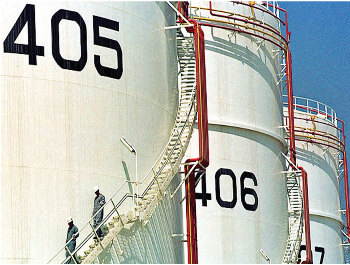
Oil reserves storage tanks in UAE
