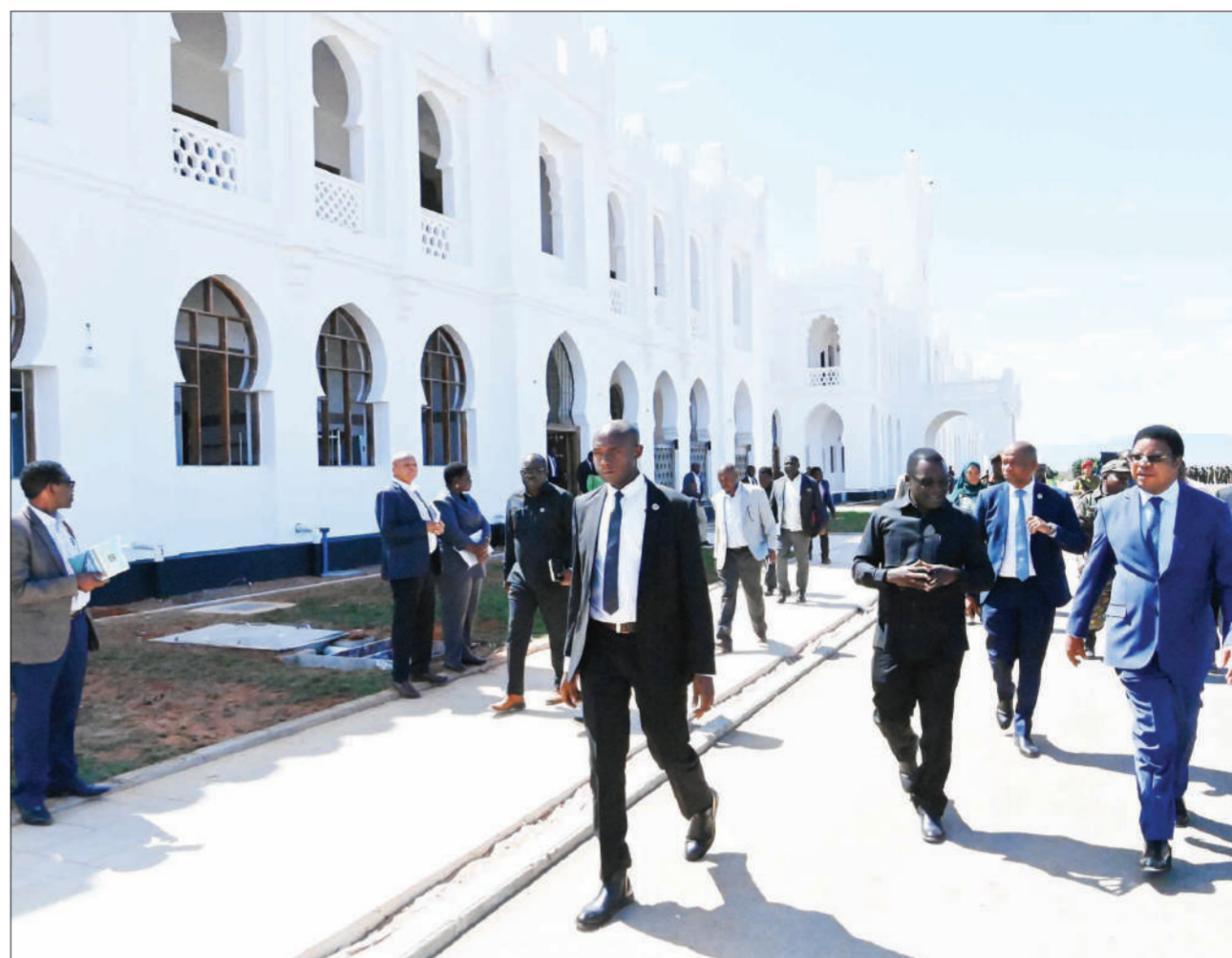
Prime Minister Kassim Majaliwa has an eyewitness account yesterday of progress in on-going construction at Chamwino State House in Dodoma. Photo: PMO
