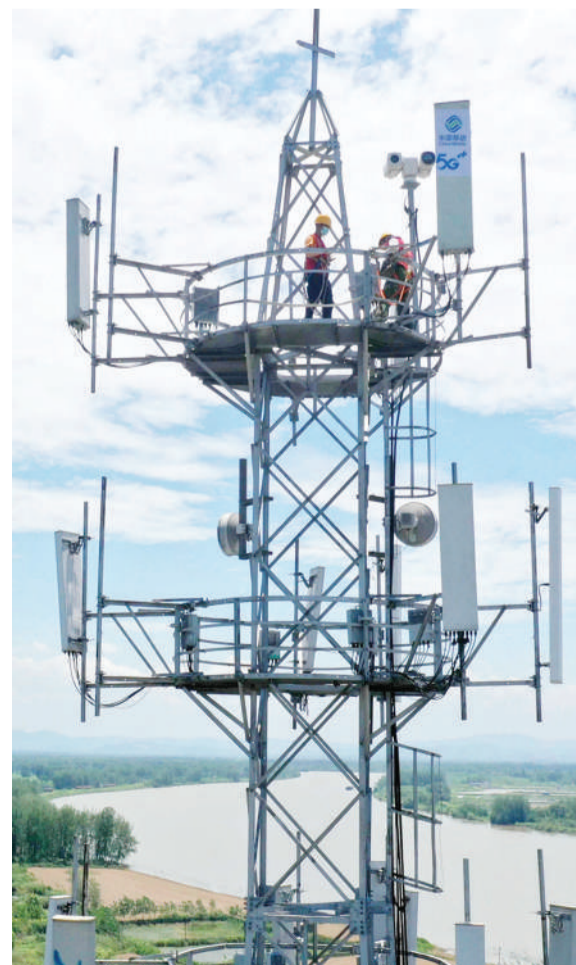
Photo taken on July 8, 2022 shows workers adjusting antennas at a 5G base station in Xuba township, Tongling, east China's Anhui province. (Photo by Guo Shining/People's Daily Online)
