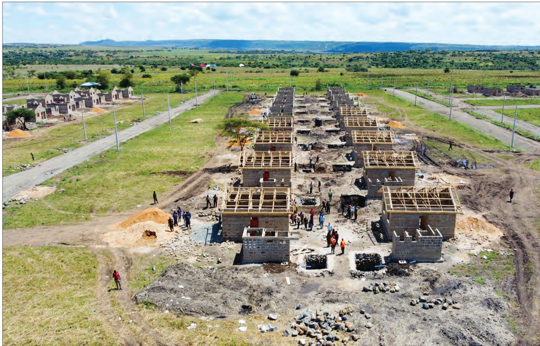
This is an aerial view of some of the houses being built at Waret in Hanang District, Manyara Region, for victims of the mudslides that hit the area in December last year. The scene was captured yesterday. Photo: PMO
