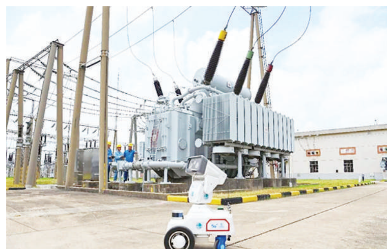
A 5G-enabled intelligent robot conducts routine inspection of electrical equipment at a 220kV substation in Dingyuan county, Chuzhou, east China's Anhui province. (Photo by Song Weixing/People's Daily Online)
