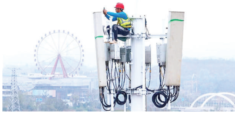
A mobile telecommunication technician tests 5G network on a 5G base station in Ganzhou, east China's Jiangxi province. (Photo by Zhu Haipeng/People's Daily Online)
