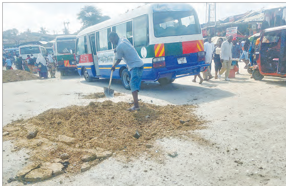
A Dar es Salaam resident patches potholes at Mbezi Mwisho bus terminal in the city yesterday to address inconvenience to commuter bus drivers. Photo: Correspondent Sabato Kasika
