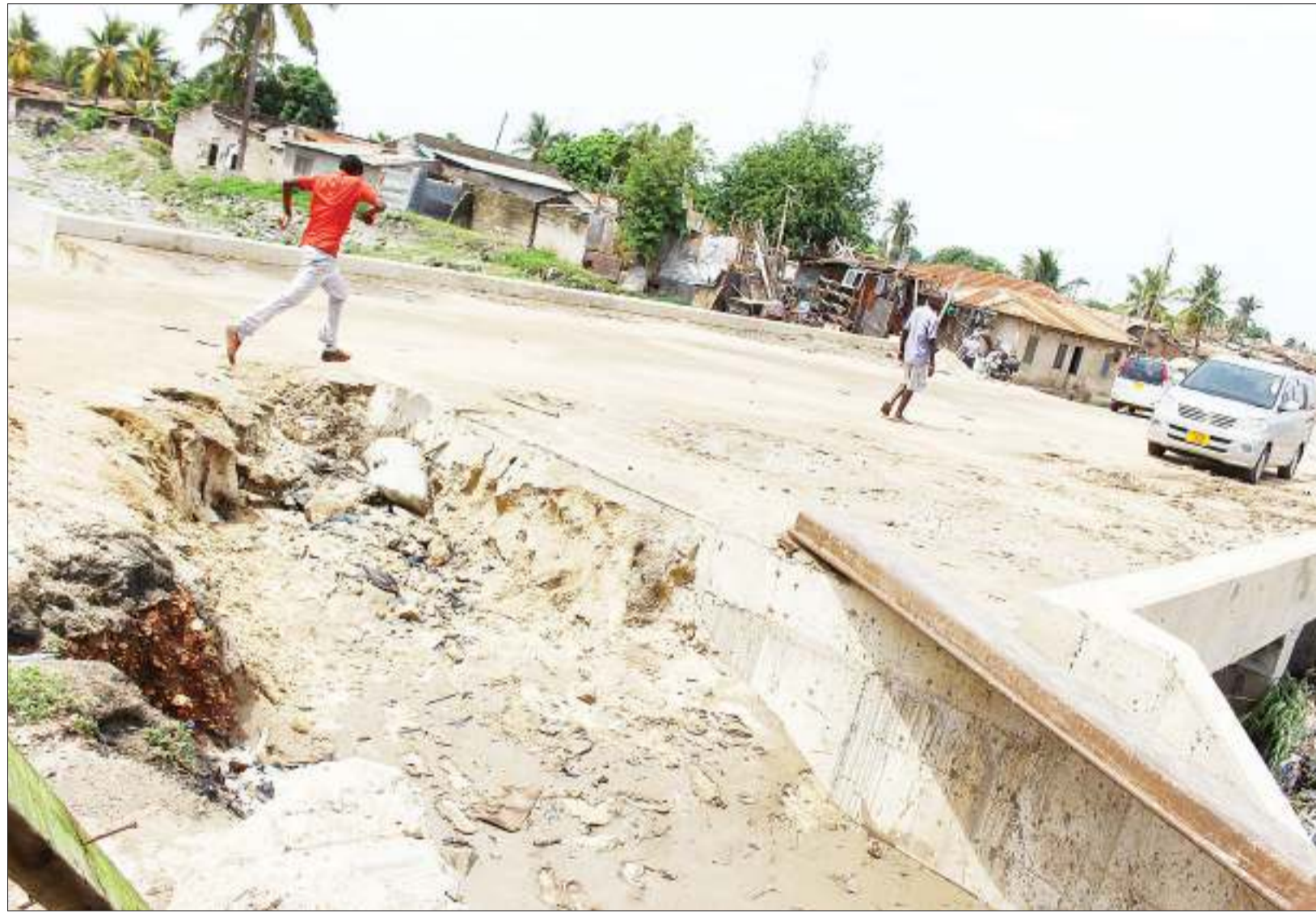
A Dar es Salaam resident finds no option at the weekend but to demonstrate his long jump prowess in crossing a newly built bridge on the road linking Dar es Salaam's Tandale and Mwananyamala kwa Manjunju suburbs which has already been damaged by rain and calls for urgent rehabilitation. Photo: Halima Kambi
