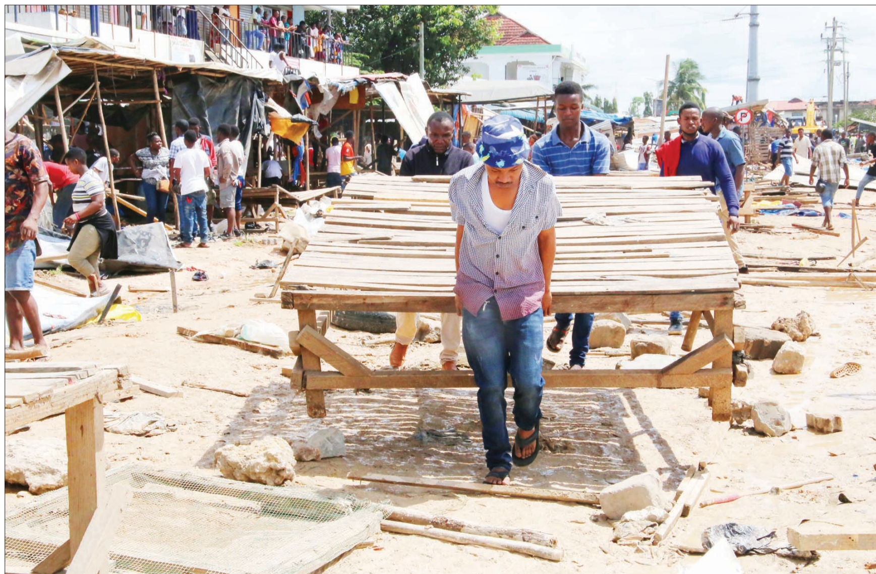
Small traders at Mwenge, Dar es Salaam, relocate yesterday to pave the way for the expansion of a five-km stretch of Ali Hassan Mwinyi Road, a project to be implemented from Morocco to Mwenge by a Japanese contracting firm. Photo: Selemahni Mpochi
