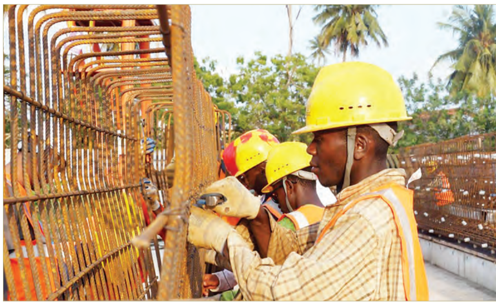
Workers bind prefabricated beam reinforcement at a construction site of an interchange, part of a project to rehabilitate and improve 100 kilometers of roads in Zanzibar, Tanzania, taken by China Civil Engineering Construction Corporation (CCECC). (Photo by Wang Di/People's Daily)
