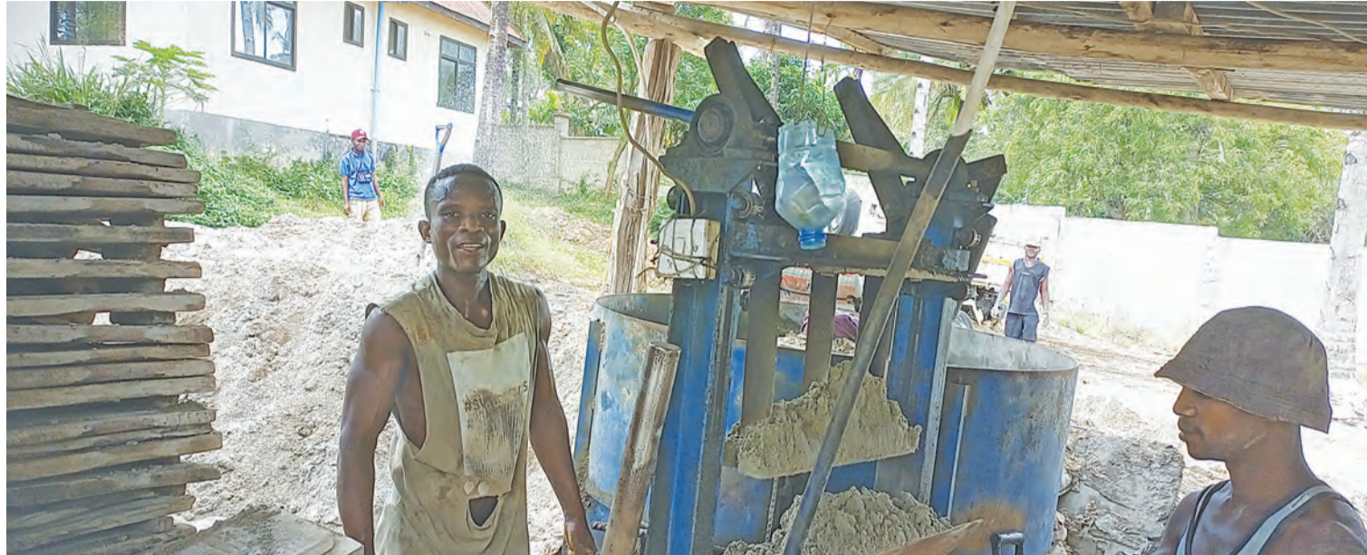
Moses Mwingwa (38) (R) works as a mortar operator without protective gear. Assisting him is Erasto Kubindi (41). Photo: Francis Kajubi.
