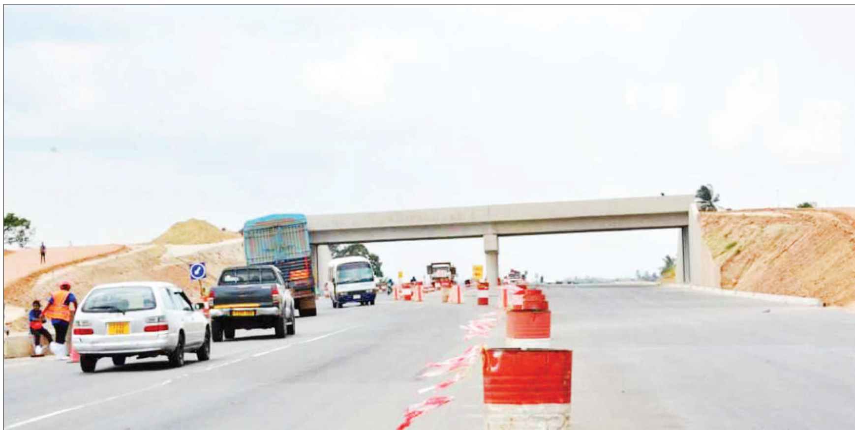
This is Kibamba overhead bridge near Mloganzila in suburban Dar es Salaam, as captured by Correspondent Miraji Msala yesterday. It constitutes part of the first phase of the widening of the 19-km stretch of Morogoro Road from Kimara to Kibaha into a six-lane dual carriageway, including the construction of three bridges - at Kibamba, Kiluvya and Mpiji.
