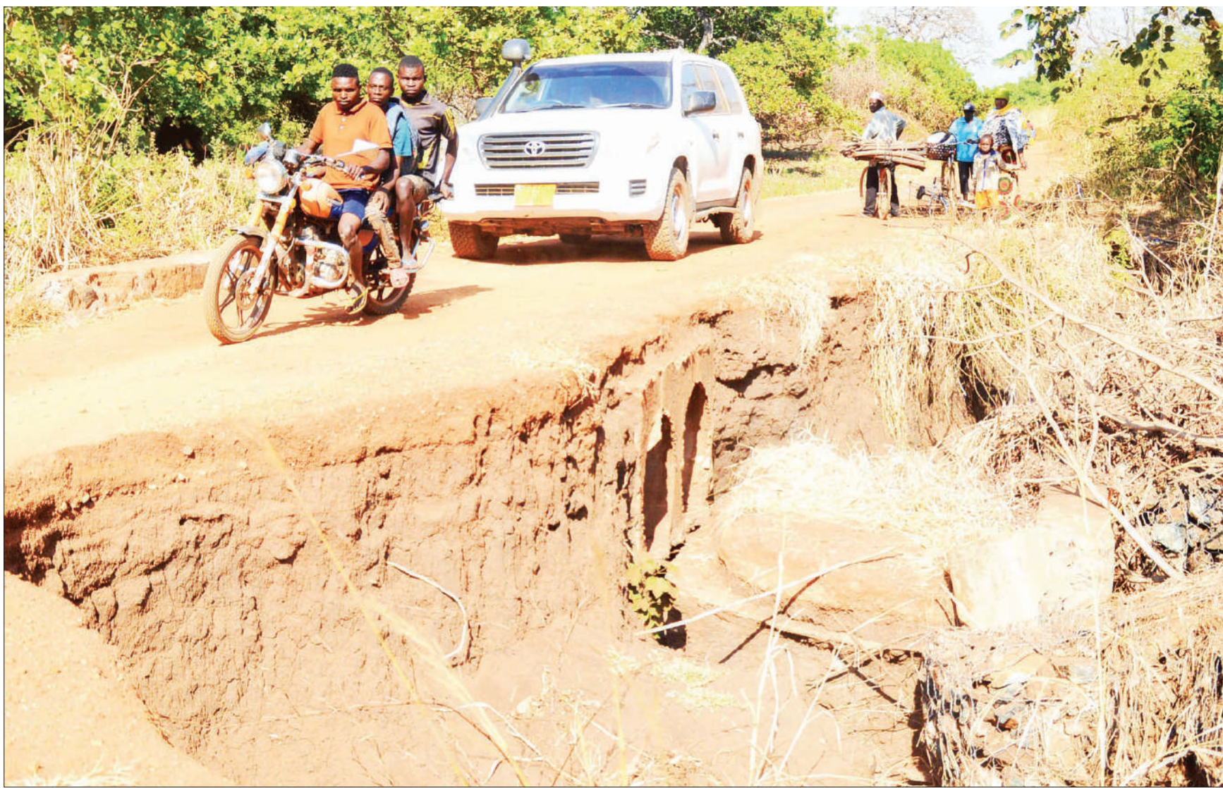
Motorists find the going challenging along a damaged stretch of the Nachingwea-Ruangwa road in Lindi Region, as found on Thursday. This is at Kipara village in Mnero ward in Nachingwea District. Photo: Correspondent Said Powa
