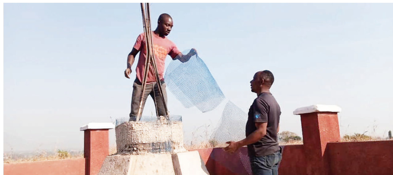
Contractors pictured working at Kola cemetery's memorial tower in Morogoro recently. Morogoro District Commissioner, Bakari Msulwa, had ordered the project worth 18m/- must be completed this weekend. The tower is expected to be among the region's tourist attractions as it will provide details on people, who lost their lives in a fuel tanker explosion in the region last year. PHOTO: MICHAEL SIKAPUNDWA
