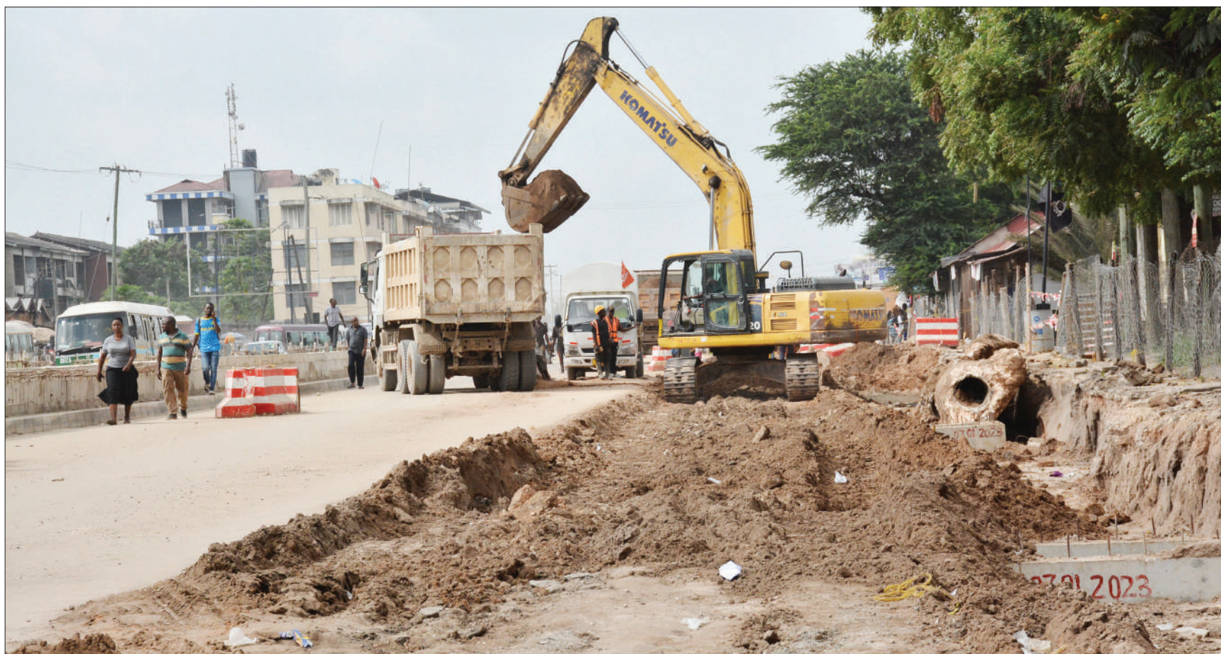
Dar es Salaam Rapid Transit (DART) Project Phase III construction of the 23.6 kms stretch from the Nyerere-Gongolamboto Road to the Central Business District is progressing well at Buguruni area as captured by our roving photographer yesterday. Photo: Correspondent Miraji Msala
