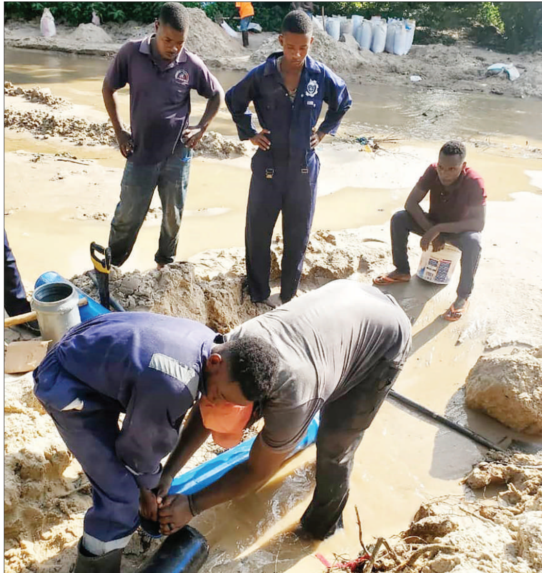
Technicians with the Dar es Salaam Water and Sanitation Authority (DAWASA) continue with the maintenance work of laying pipes at Gwajima Salasala Bridge following heavy rains recently. Photo: Correspondent Joseph Mwendapole
