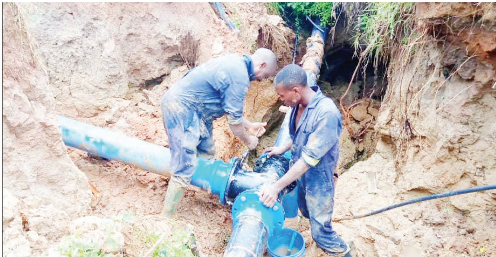
Dar es Salaam Water and Sanitation Authority technicians work on a pipe meant to supply water to Tatedo and National Examinations Council of Tanzania premises, Mbezi Juu and several other parts of the city, as captured yesterday. Photo: Guardian Correspondent
