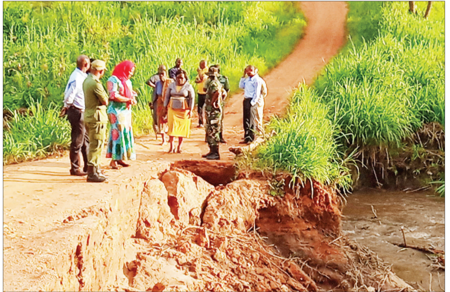
Kilolo District Commissioner Asia Abdallah (2nd L) and Defence and Security Committee members inspect Malafu ward bridge which had been swept away by floodwaters yesterday. Photo: Correspondent Francis Godwin
