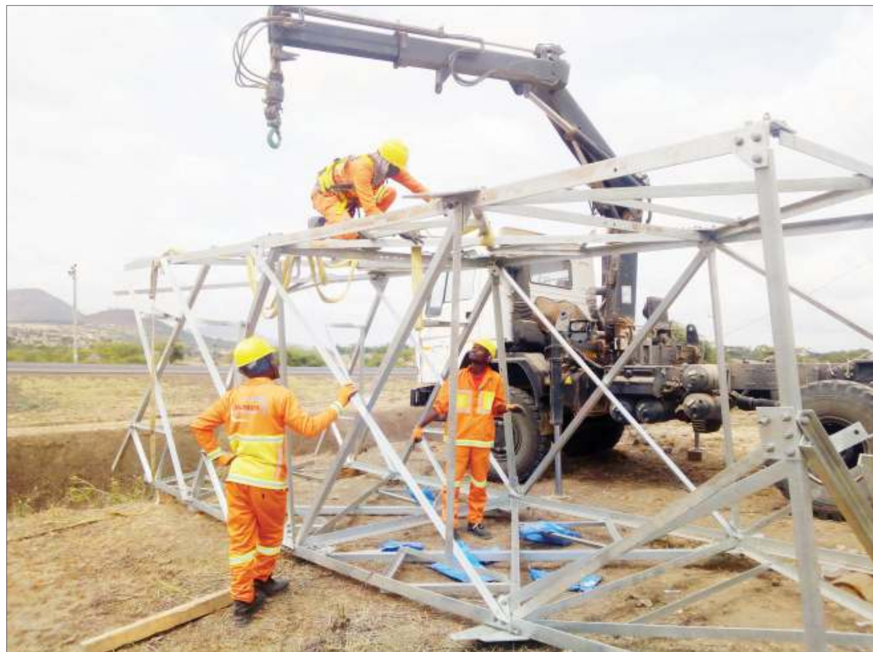
Booygues Energies & Services technicians assemble a high-tension steel-reinforced power tower for the 400-KV Kenya-Tanzania Power Interconnection project at Kisongo area in Arusha yesterday. The electricity lines will run from Singida to the Namanga border post via Babati and Arusha. Photo: Correspondent Woinde Shizza
