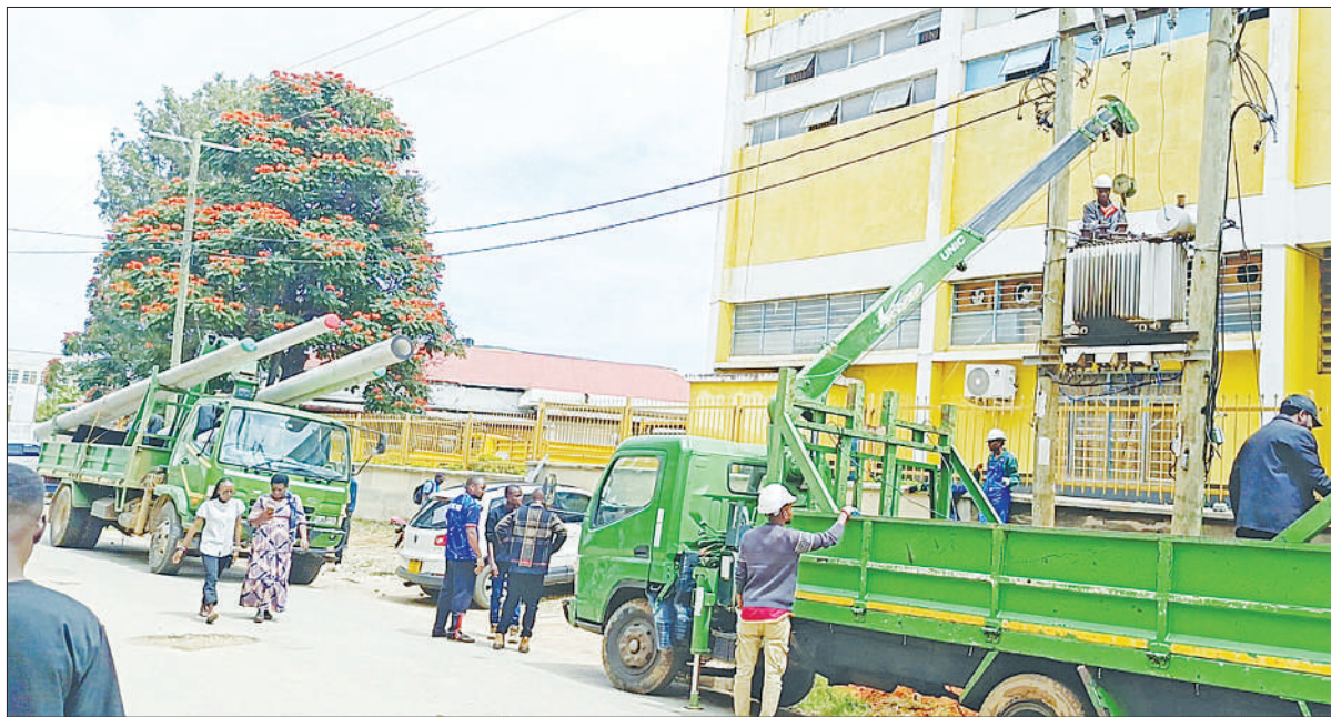
Tanzania Electric Supply Company (TANESCO) technicians install a high voltage capacity transformer and replace wooden poles with concrete ones at Miyomboni area in Iringa Municipality at the weekend. Photo: Correspondent Francis Godwin
