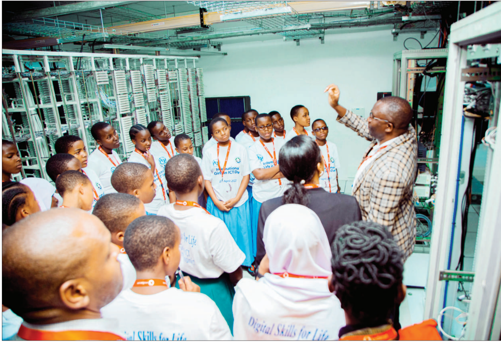
Josiah Kizinda (R), Vodacom Tanzania's Dodoma Data Centre maintenance manager, pictured in the national capital at the weekend briefing 96 female students from some secondary schools in the Central zone region on the operations of the machines used at the centre. The students were on a study tour coordinated by Universal Communications Service Access Fund (UCSAF) and meant to sensitise female students into pursuing science and ICT courses under the 'Girls in ICT' project implemented in partnership with the Tanzanian government. Photo: Guardian Correspondent
