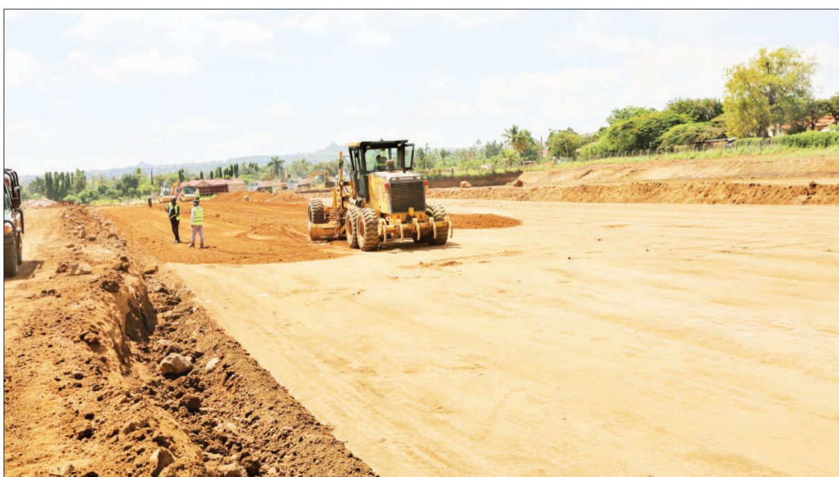
A grader levels unpaved runways at Musoma airport in Mara region which is under construction at tarmac level yesterday. Photo: Guardian Correspondent
