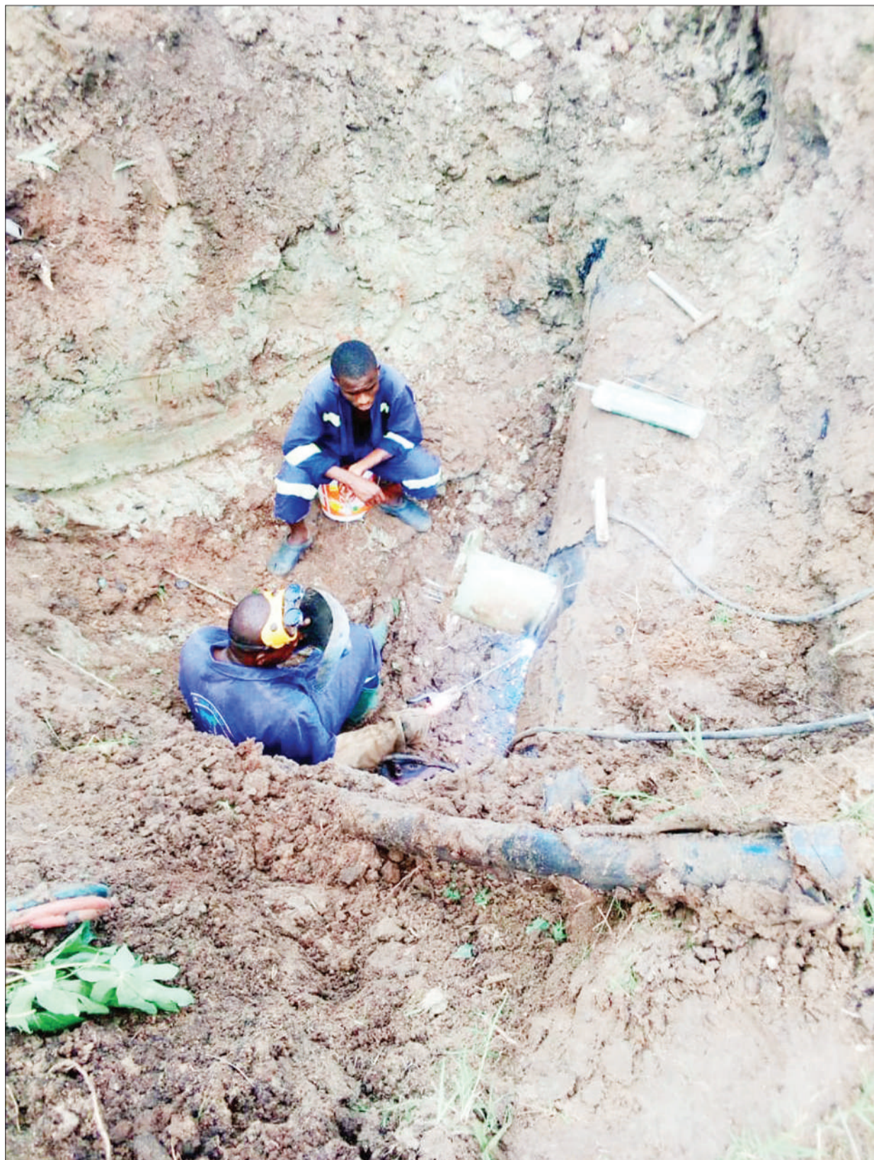
Dar es Salaam Water and Sanitation Authority (Dawasa) technicians move to repair a leaking pipe in the Luguruni suburb yesterday. Photo: Guardian Correspondent
