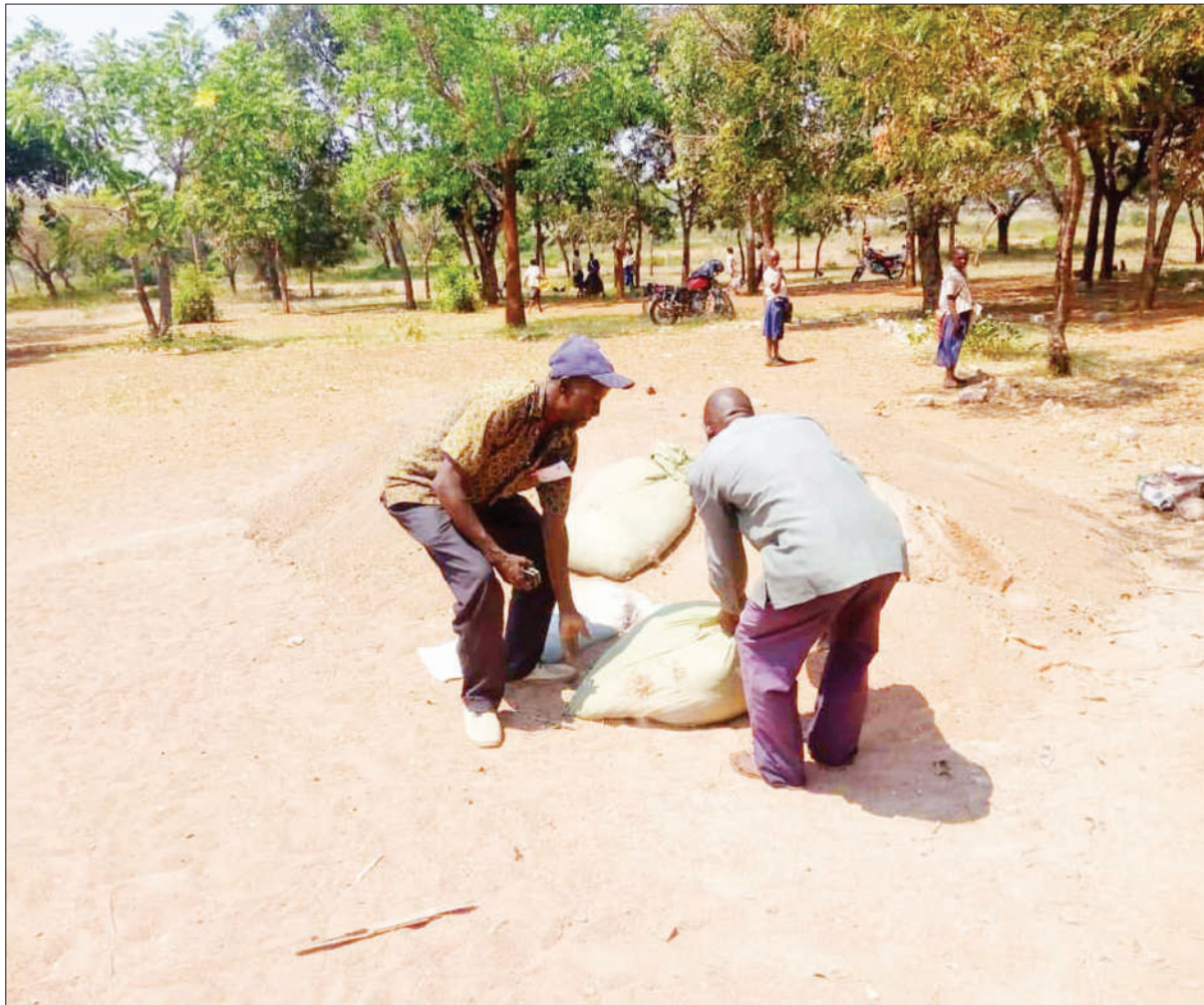
Benjamin Lazaro (L) and Majira Makoba, locality leaders at Kakisheri village in Musoma Rural constituency's Nyakatende ward, pictured at the weekend collecting sand for use in the construction of classrooms and a teachers' house for Kambarage Primary School. Photo: Guardian Correspondent
