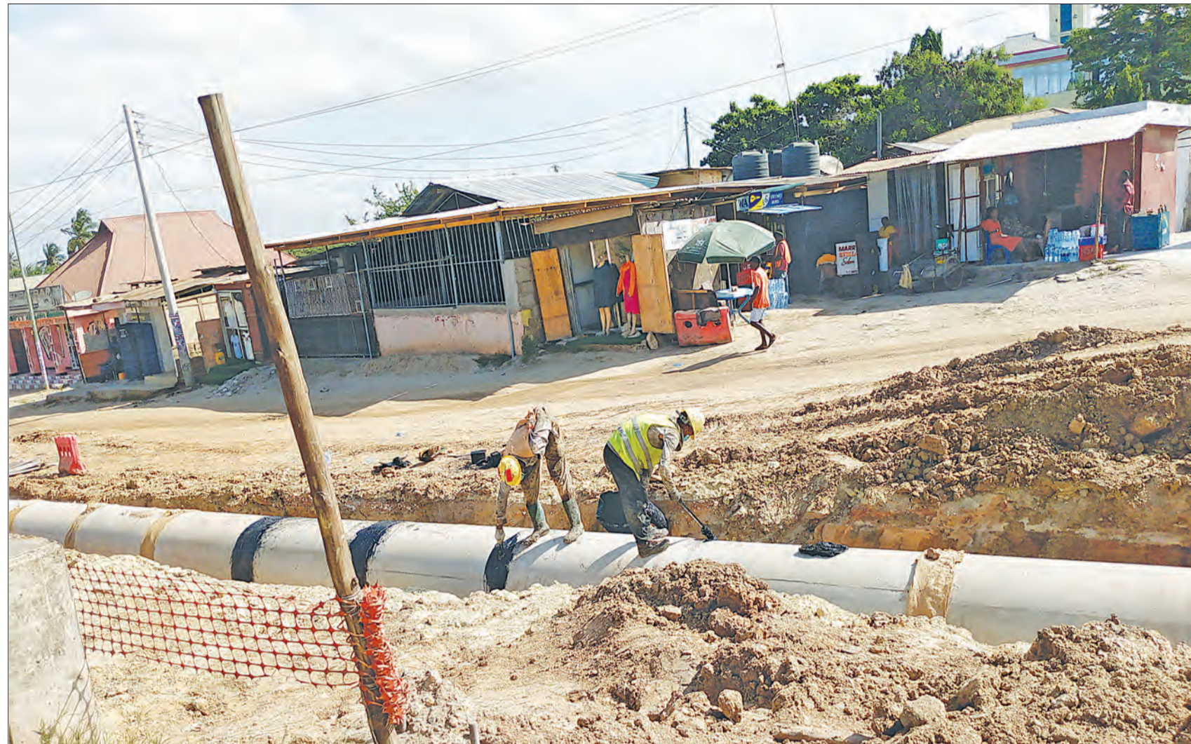
Work on storm water drainage infrastructure well in progress yesterday along the Kimara-Korogwe stretch of Dar es Salaam's Morogoro Road, which is undergoing expansion. Photo: Correspondent Sabato Kasika
