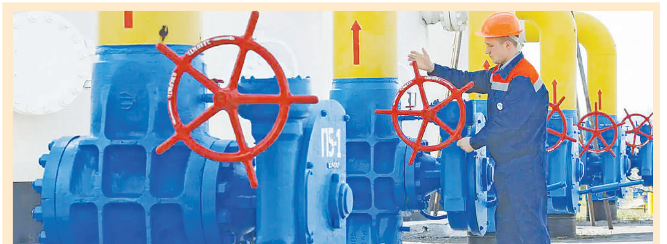
Russia gas facility
