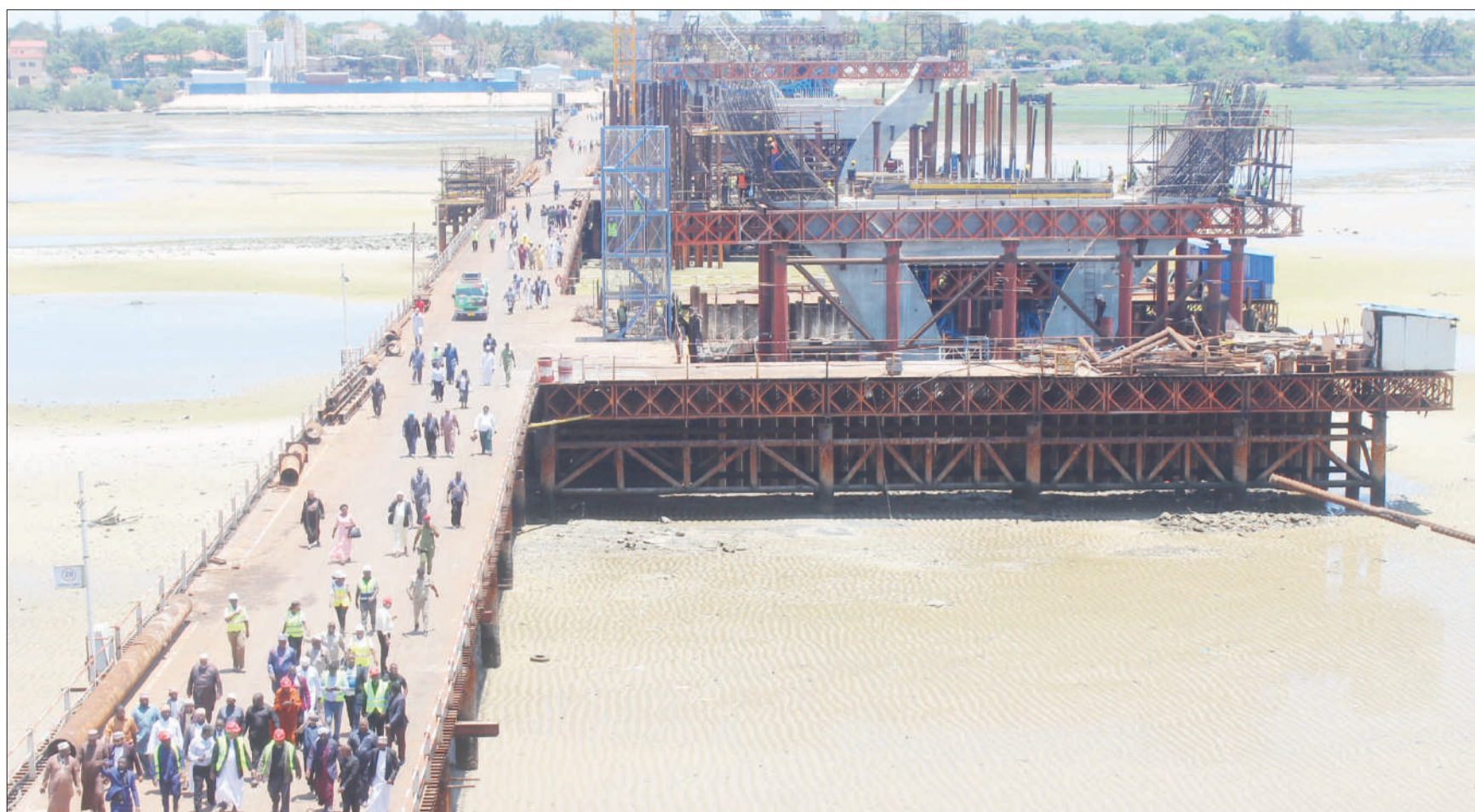
This is a scene from the site of the ongoing construction of Dar es Salaam city's 6.3-km Tanzanite Bridge, which is meant to link the Aga Khan Hospital section of Upanga East and Coco Beach/Oysterbay via India Ocean waters, as captured yesterday. Photo: Correspondent Jumanne Juma
