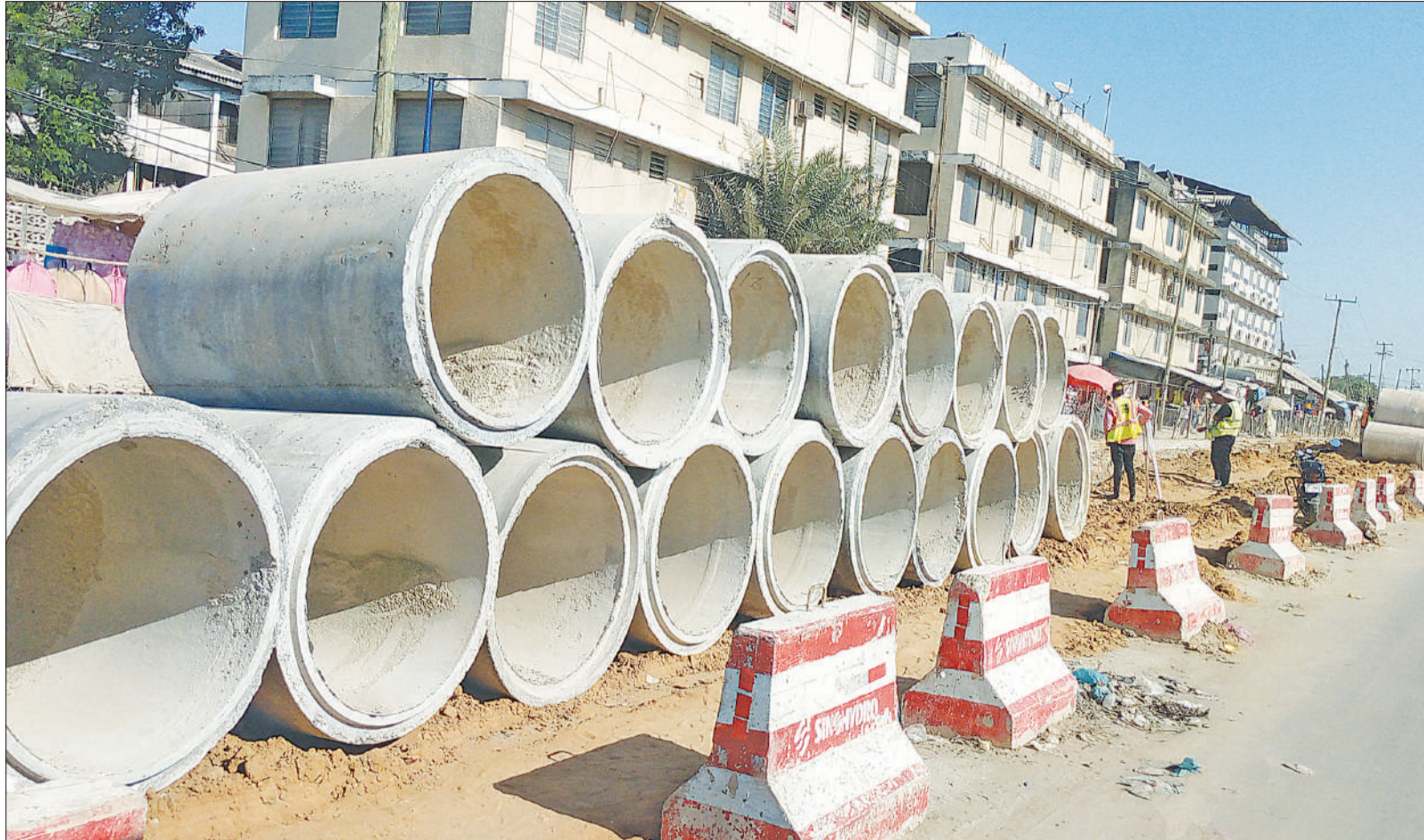
Culverts lined up at a Buguruni section of Dar es Salaam's Uhuru Street on Monday awaiting use in the ongoing construction of infrastructure for the city's rapid transit bus project. Photo: Correspondent Sabato Kasika
