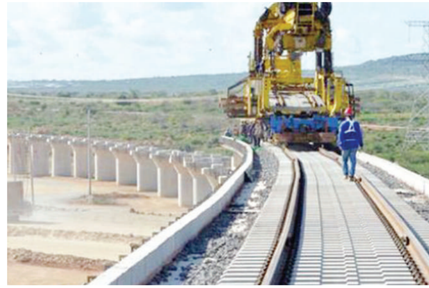
Ongoing construction of the Standard Gauge Railway (SGR) network in Tanzania. The Value of construction sector is expected to hit 30trn/- by 2026 PHOTO/FILE
