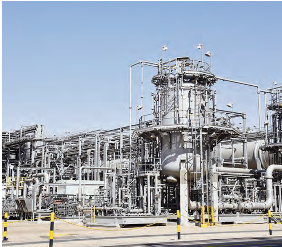
Photo taken on June 28, 2021 shows the industrial estate of Saudi oil giant Aramco in Dammam, Saudi Arabia. (Xinhua/Hu Guan)
