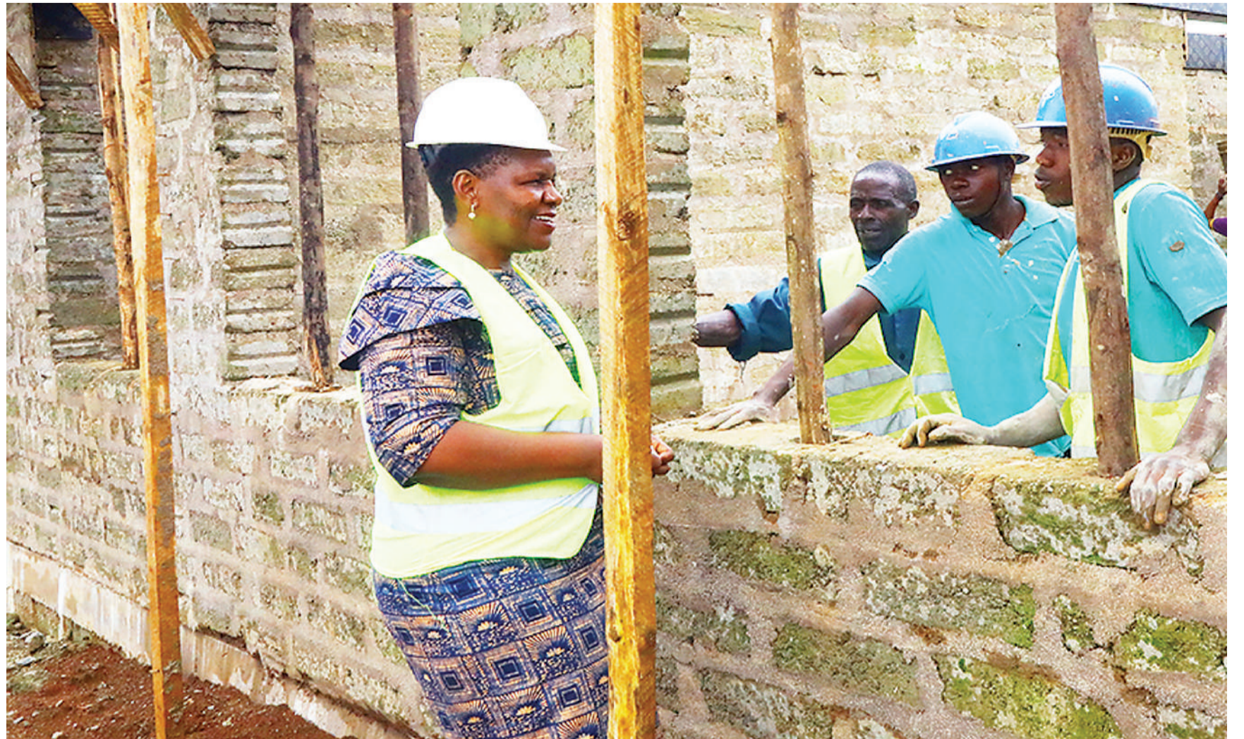
Deputy minister for Land, Housing and Human Settlements Development, Dr Angeline Mabula (L) inspects the ongoing construction of Tanzania Forest Services (TFS) office building being undertaken by the National Housing Corporation (NHC) at Iyondo Msimwa forest farm in Ileje district, Songwe region this week. Photo: Correspondent Munir Shemweta
