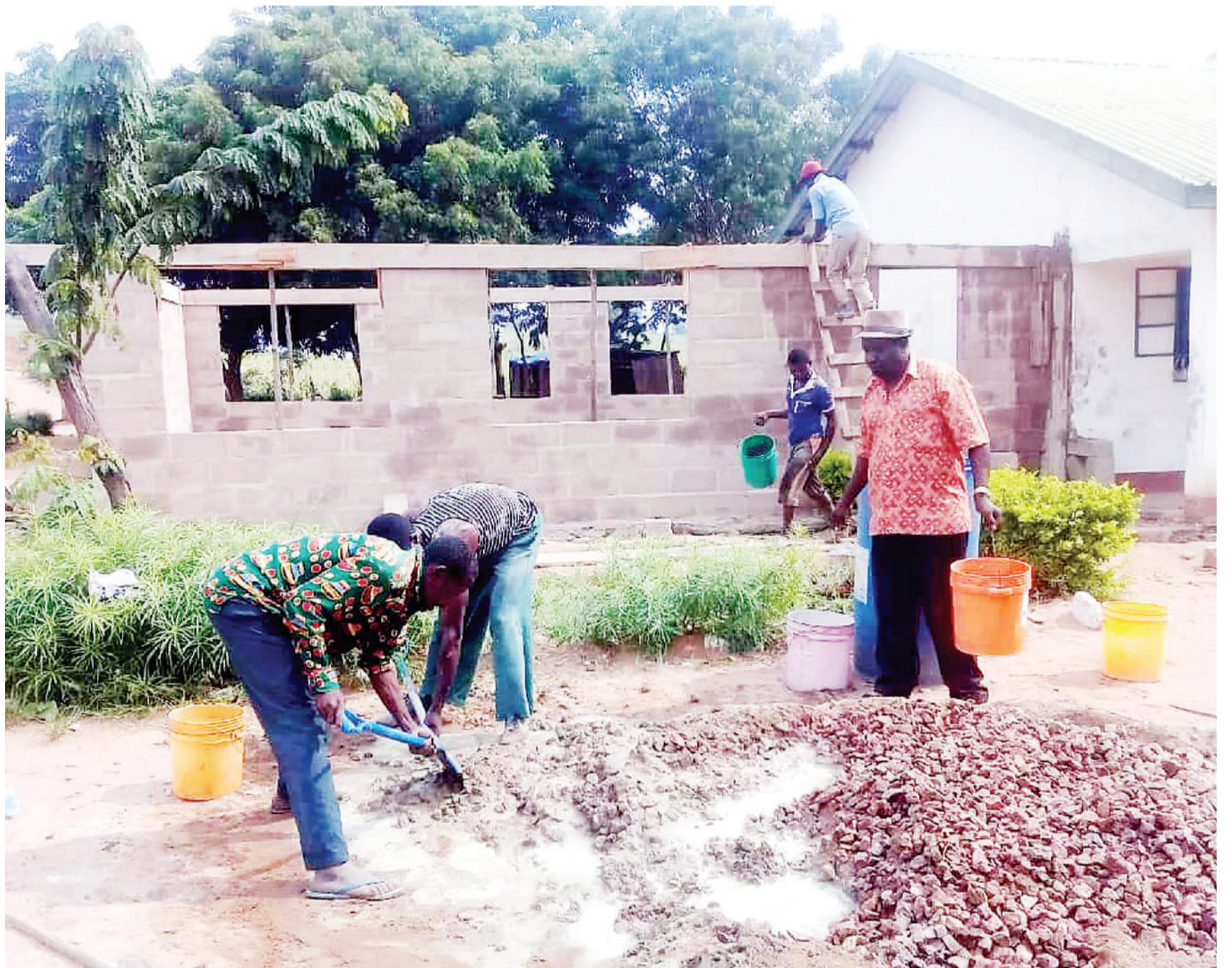
Technicians at the construction site of one of classrooms for first-year students at Rusoli ward secondary school in Musoma rural, Mara region this week. The schools had already enrolled a total of 132 students. Photo: Guardian Correspondent
