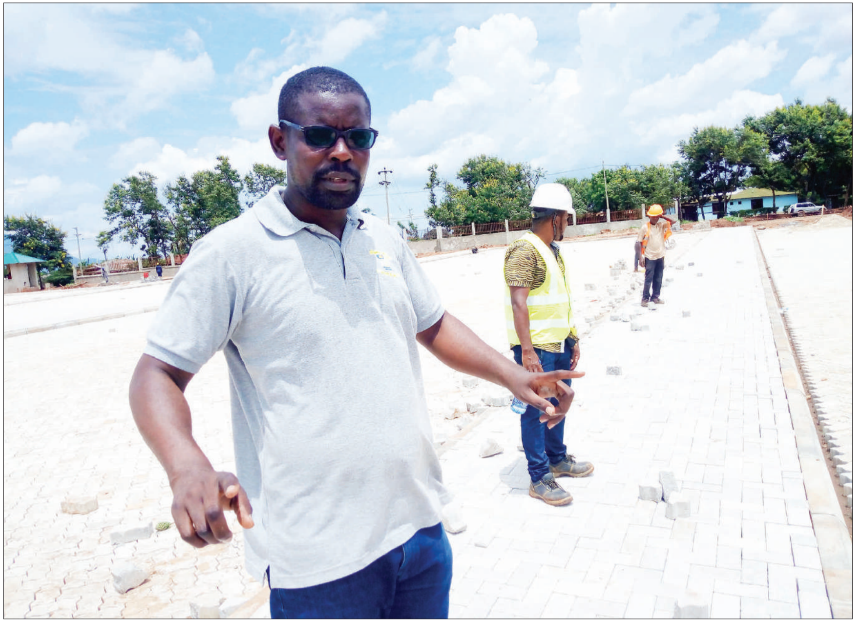
Mnene James, Urban Local Government Strengthening Programme manager for Morogoro, remarks on the ongoing construction of the municipality's modern commuter bus stands construction at Mafiga. The work began on May 10, 2019 and is lined up for completion this May, with Nandahra Engineering and construction Co. Ltd as the contractor. The first phase, which is expected to cost 14bn/-, will enable the accommodation of 40 taxis, 32 tricycles and 23 motorcycles as well as provide parking lots for 150 vehicles at a go. Photo: Correspondent Michael Sikapundwa
