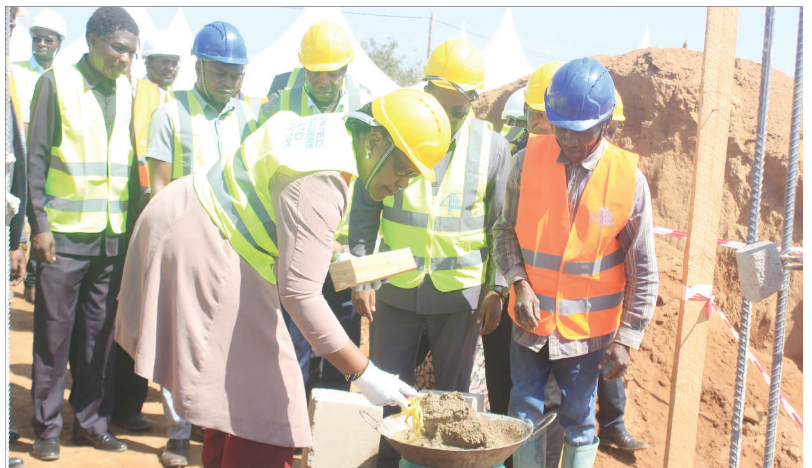
Dr Angelina Mabula (L, foreground), who doubles as Ilemela constituency legislator and Lands, Housing and Human Settlements Development minister, pictured in Ilemela District on Saturday inaugurating construction work signalling the realisation of the dream of establishing the Mwanza Campus of the Institute of Finance Management. Photo: Rose Jacob
