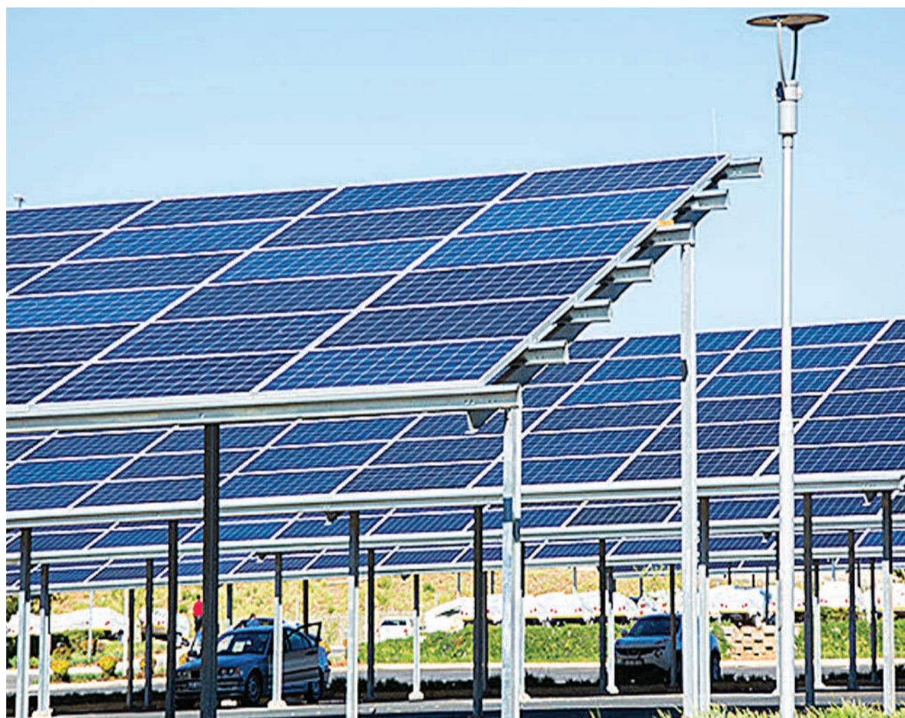
Solar panels and a model solar farm in Cape Town.
