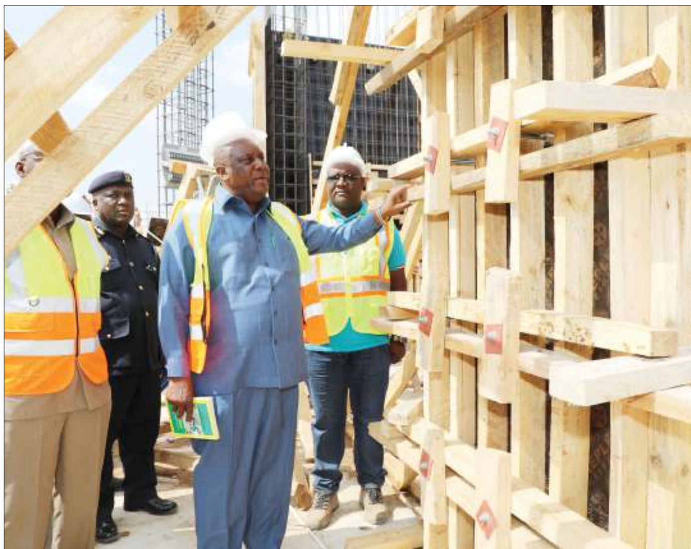
Home Affairs minister Kangi Lugola (2nd-R) has a first-hand account of the ongoing construction of the Immigration Department Headquarters building in Dodoma yesterday. Photo: Ministry of Home Affairs.
