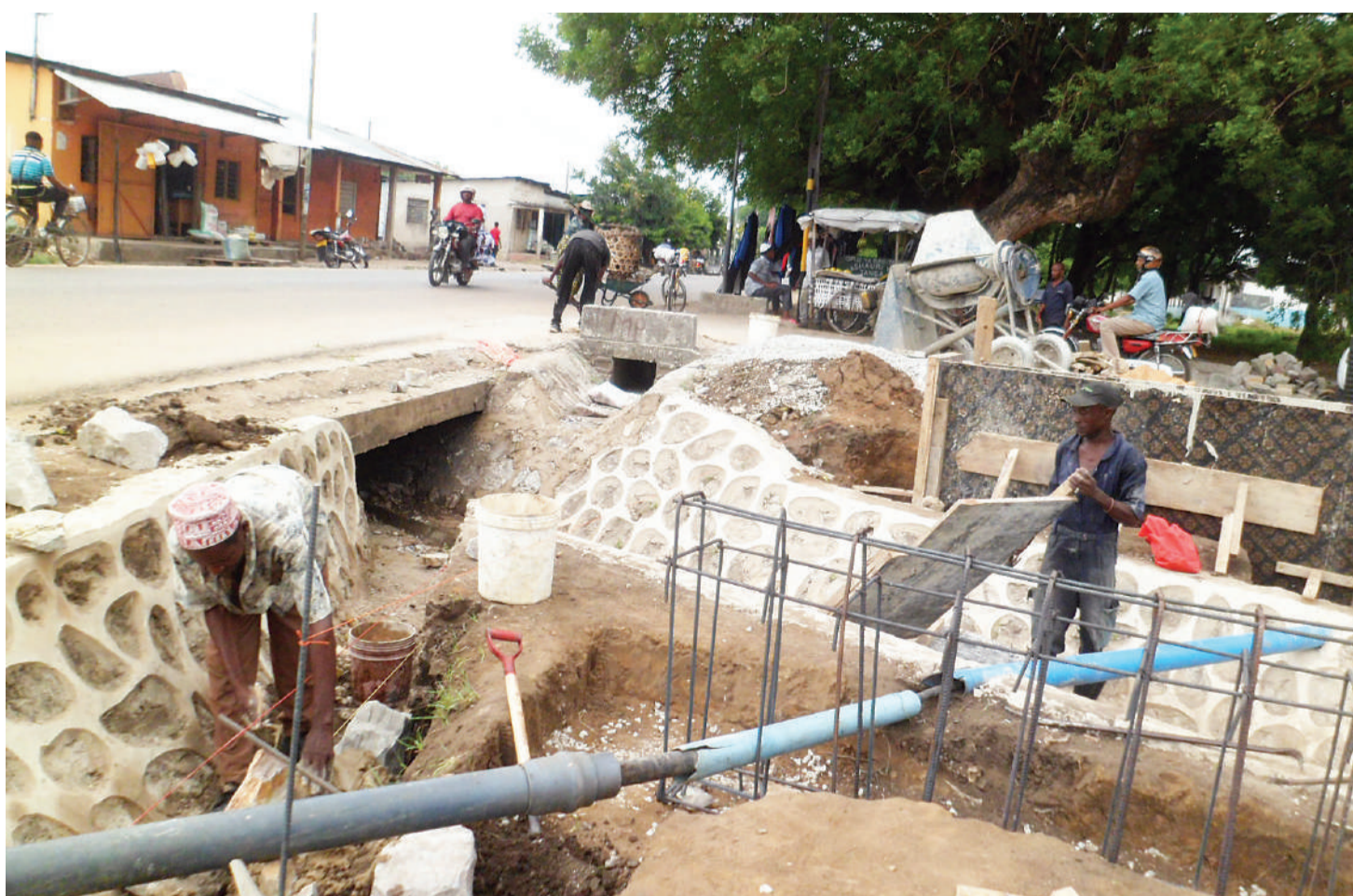
Rehabilitation of drainage system in progress at Masiwani in Tanga city's Majengo ward, as found earlier this week. Photo: Correspondent Boniface Gideon
