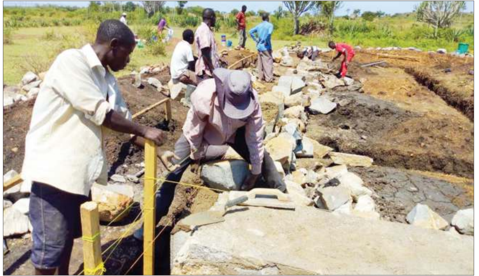
Construction of a dispensary in progress yesterday at Kakisheri village in Musoma Rural constituency's Nyakatende ward. Photo: Guardian Correspondent
