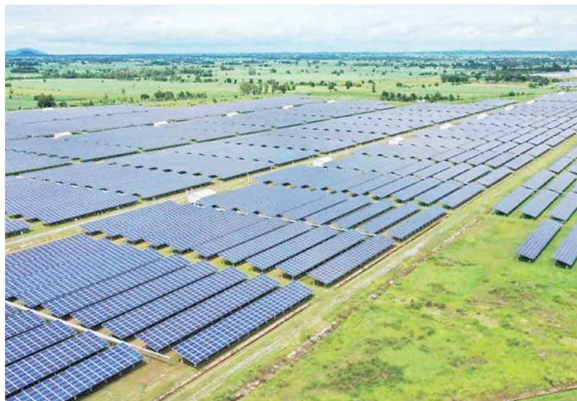
One of the solar power sites in Niger
