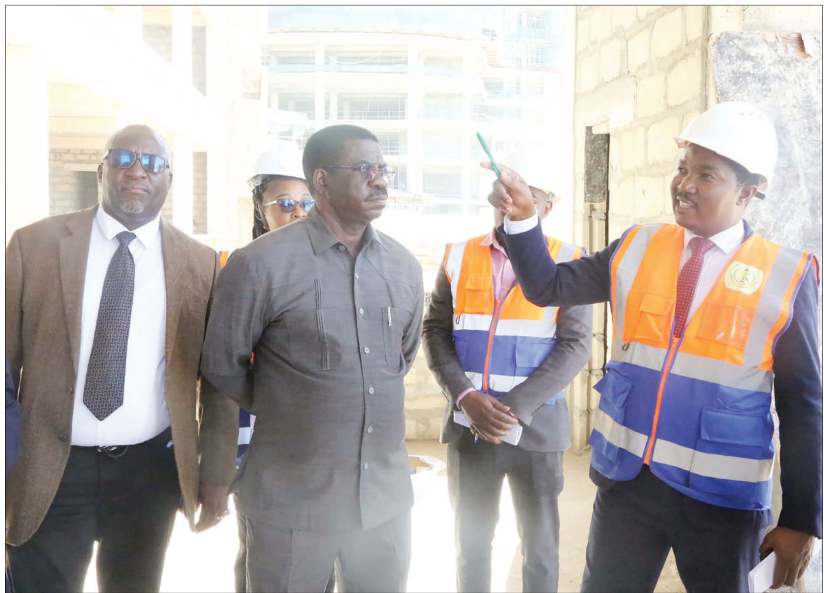
Minister of State in the Vice President's Office (Union and Environment) Dr Selemani Jafo gives orders moments after visiting the construction of Vice President's Office situated at Mtumba in Dodoma yesterday. Photo: Correspondent Robert Hokororo
