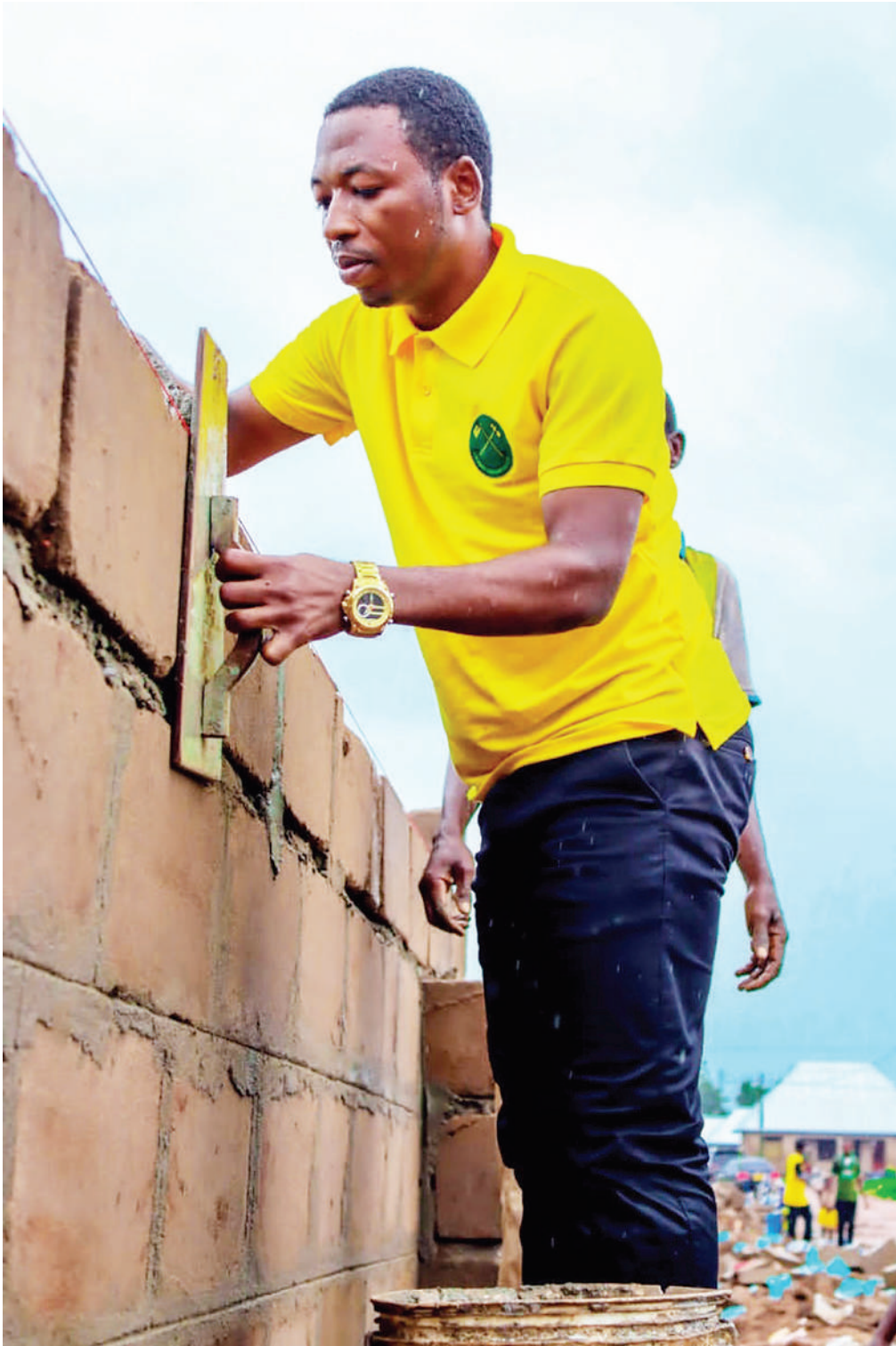
A member of the Chama Cha Mapinduzi (CCM) Youth Wing (UVCCM)'s National Council, Ramadhan Matola, participates in the construction of Kassim Majaliwa Stadium's wall in Ruangwa recently, as part of CCM's 46th anniversary celebrations which will climax on February 5. PHOTO: CORRESPONDENT
