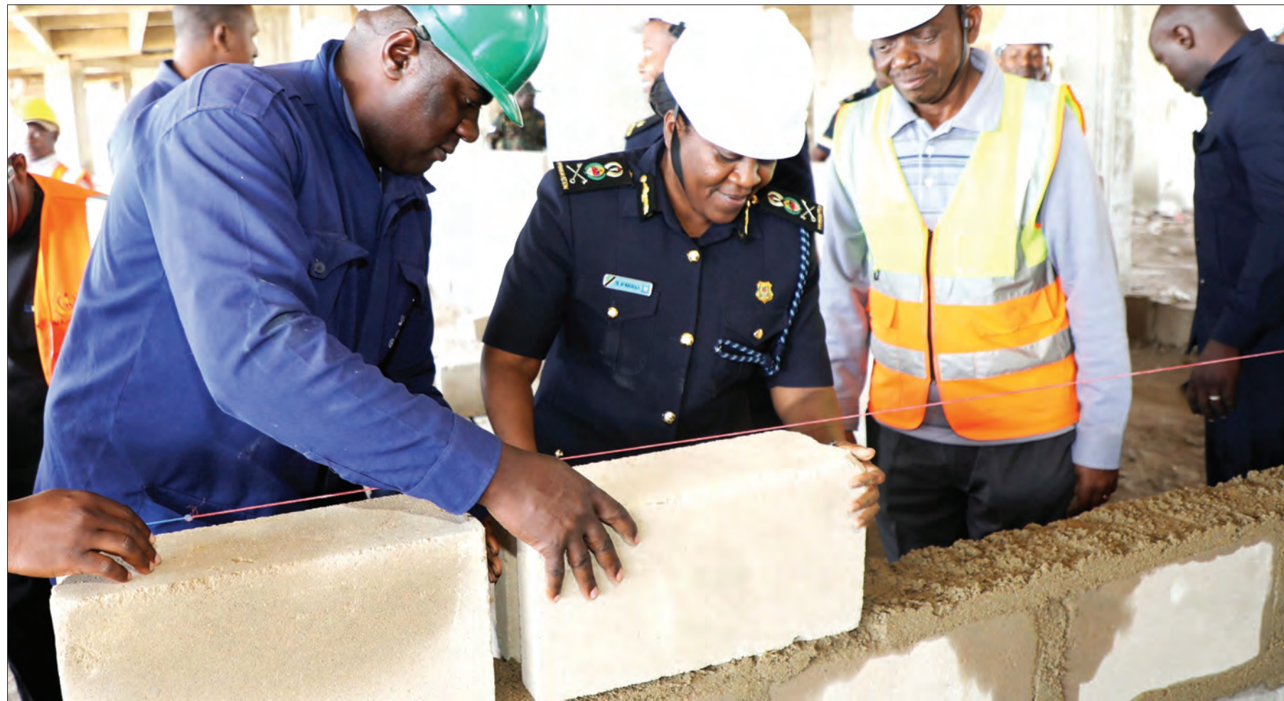
Commissioner General of Immigration Dr Anna Makakala (C) takes part in the construction of a building for the Immigration Department's headquarters in Dodoma city yesterday. Photo: Home Affairs ministry
