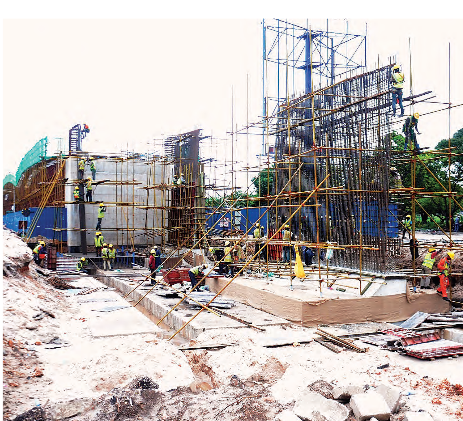
Construction of flyover at Dar es Salaam's Nyerere Road/Kawawa junction in progress, as found yesterday. Photo: Yusuph Kangabya/TUDARCO
