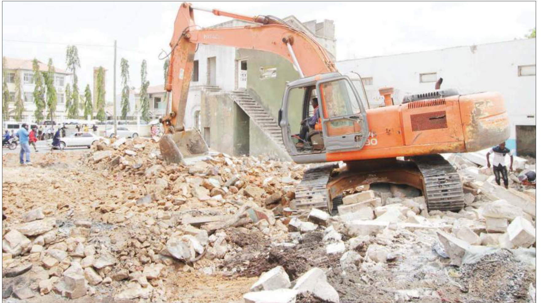
A Stecol Corporation bulldozer on a demolition mission meant to pave the way for the construction of a ten-storey commercial building at Uhindini in Dodoma city yesterday. Photo: Correspondent Ibrahim Joseph
