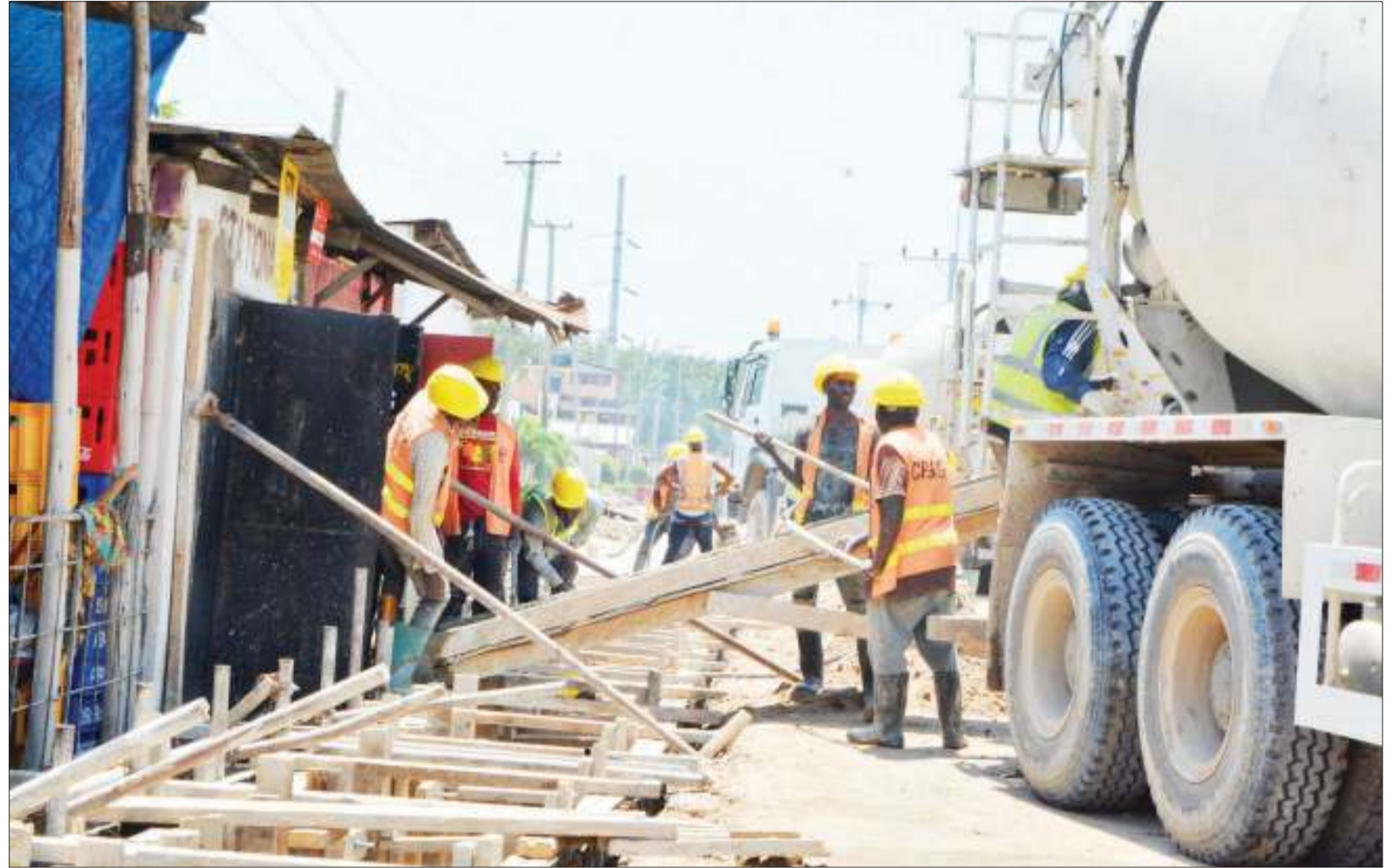
Drainage system along Salmin Amour Street in Dar es Salaam's Mwenge suburb undergoes rehabilitation yesterday. Photo: Correspondent Miraji Msala
