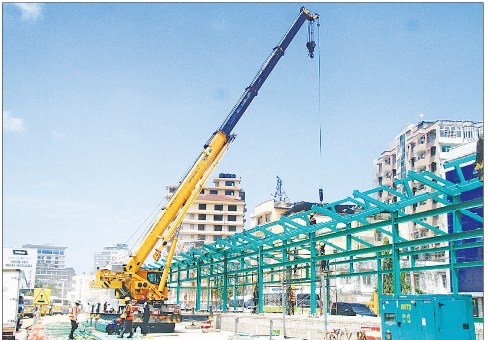
Construction of downtown Dar es Salaam's Mnazi Mmoja Bus Rapid Transit (BRT) terminal in progress yesterday. Photo: Correspondent Jumanne Juma
