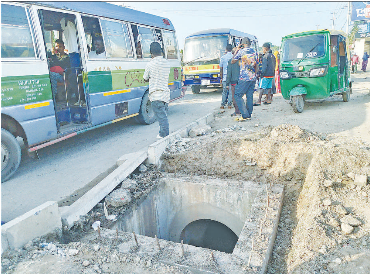
A commuter bus waits for passengers at Ukonga Banana in Dar es Salaam yesterday but, curiously, with work on open storm water drainage system far from done and putting at risk the safety of people jostling for transport. Photo: Correspondent Sabato Kasika
