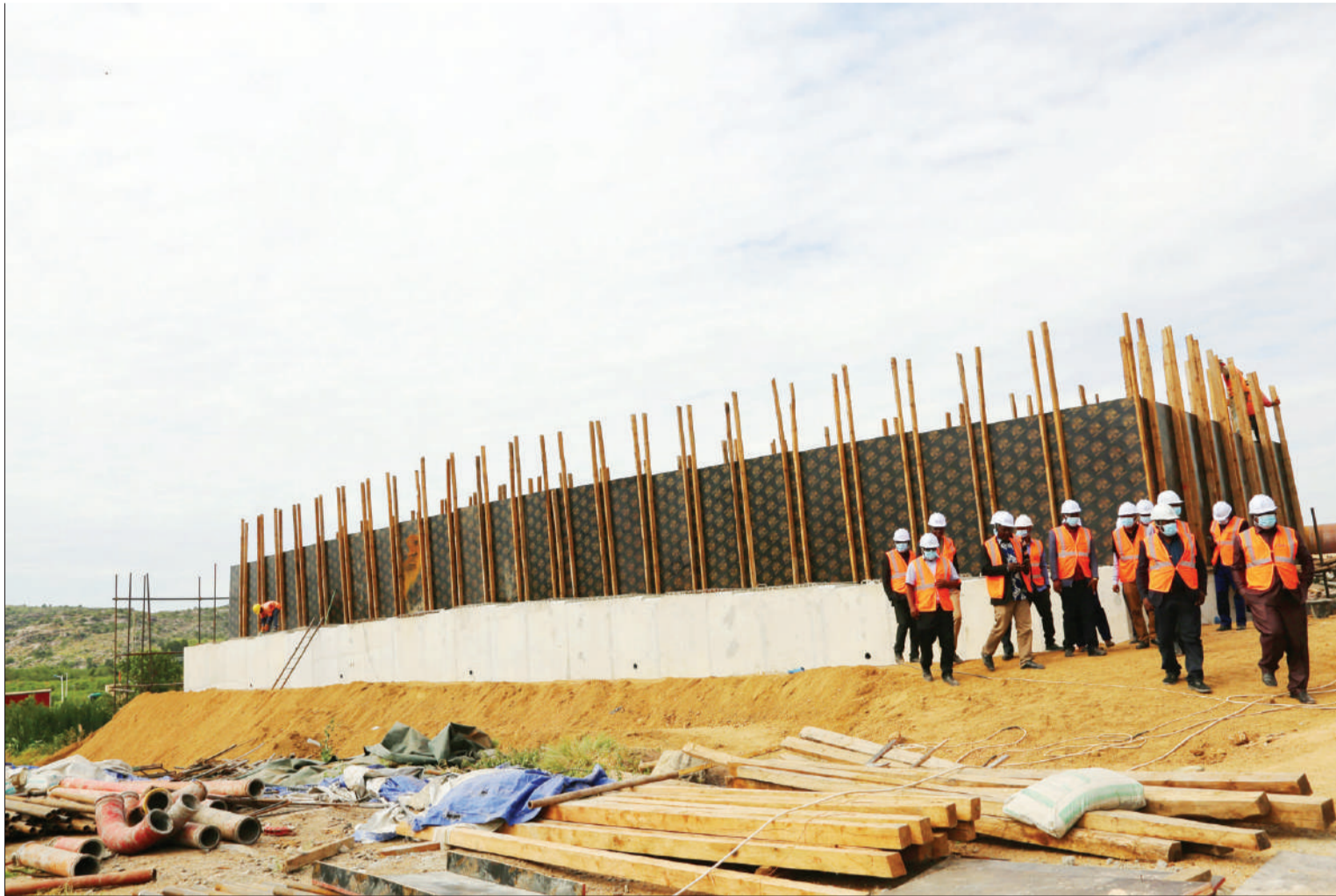
A scene at the Kigongo-Busisi Bridge, which is under construction in Mwanza Region, as captured yesterday. Photo: Guardian Correspondent
