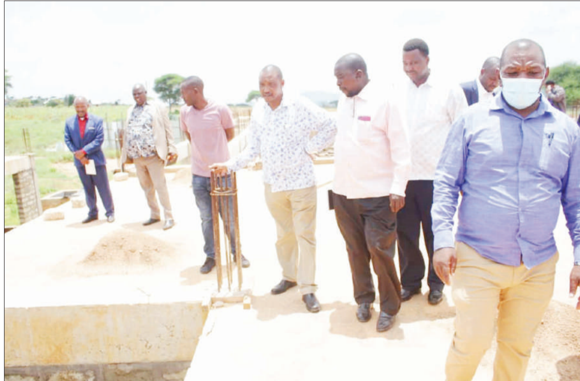
A Simanjiro District Council delegation including executive director Yefred Myenzi and chairman Baraka Kanunga pictured at the weekend assessing progress in the construction of the council's office buildings. Photo: Correspondent Gift Thadey
