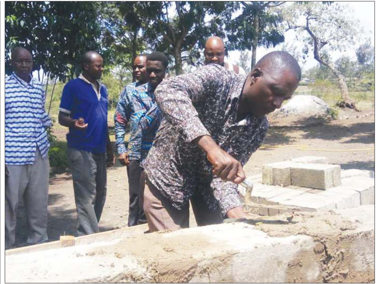
Siha district commissioner Onesmo Buswelu leads a hand in the construction of a Karansi Secondary School classroom building yesterday. Photo: Correspondent James Lanka
