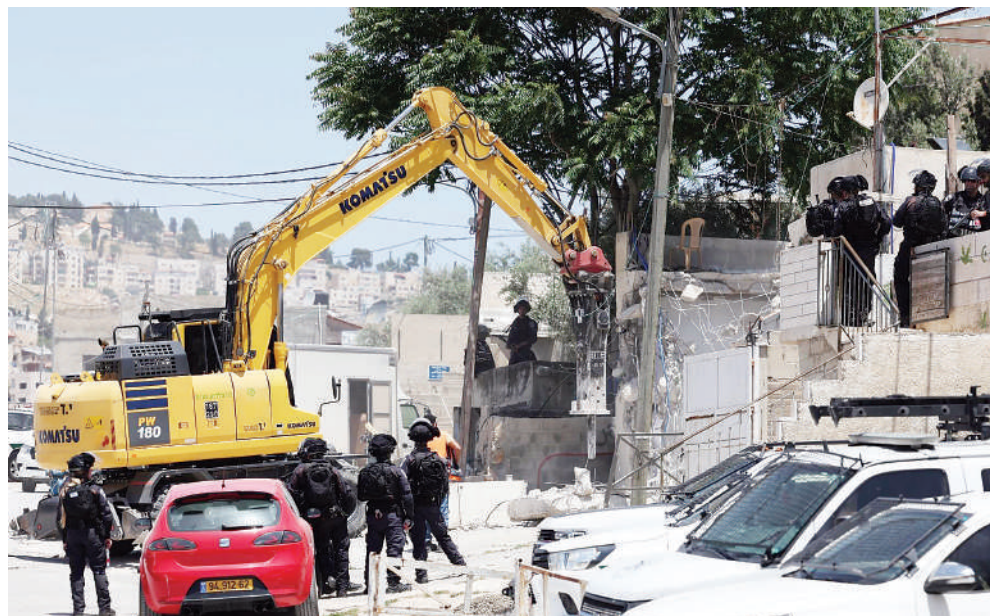
Israeli forces gather as machinery demolish a house that was built without permission in the East Jerusalem neighbourhood of Jabal Mukaber, on Monday. AFP
