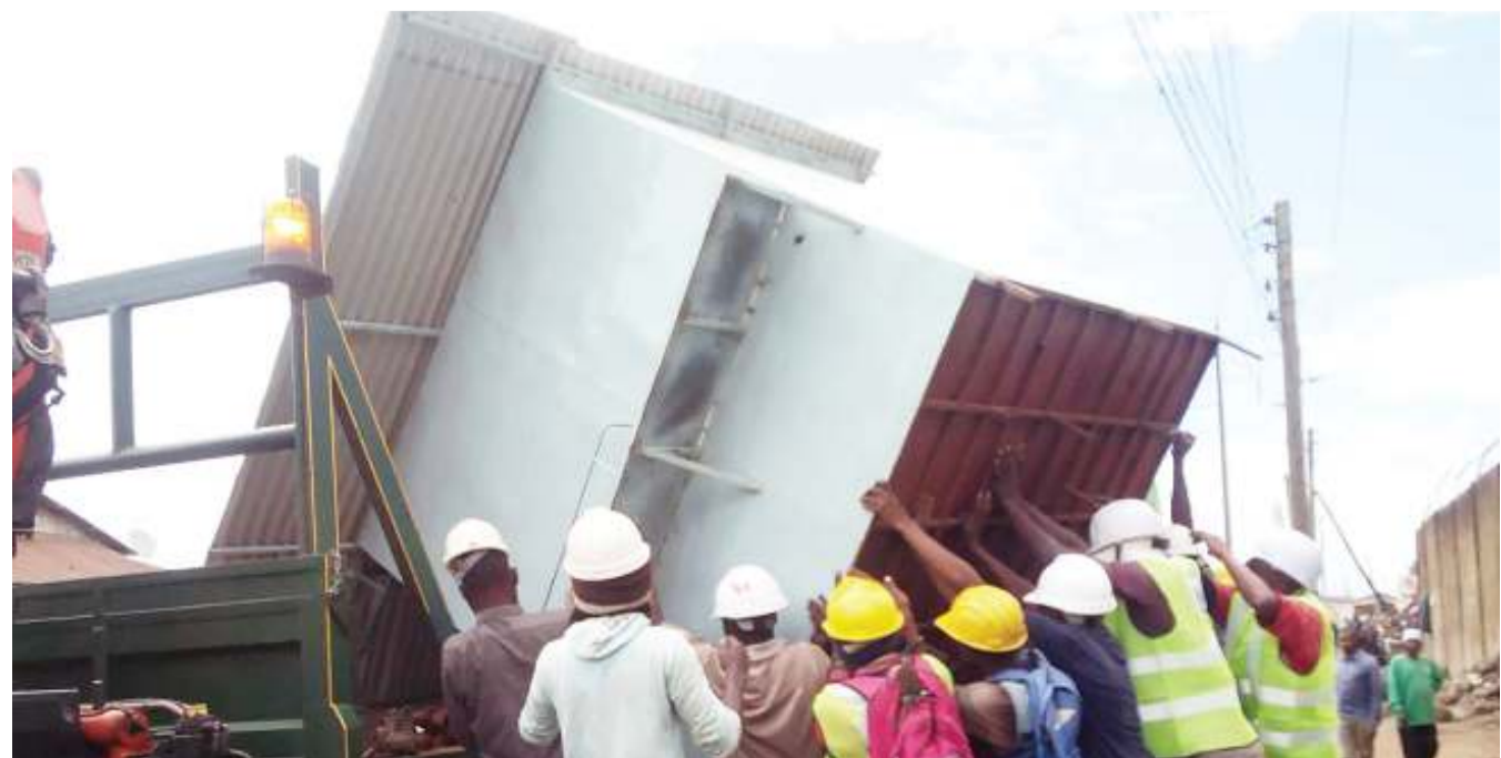
Tanzania Electric Supply Company (Tanesco) workers in Arusha pictured yesterday removing a vendor's kiosk standing right under the firm's infrastructure yesterday. Photo: Correspondent Woinde Shizza
