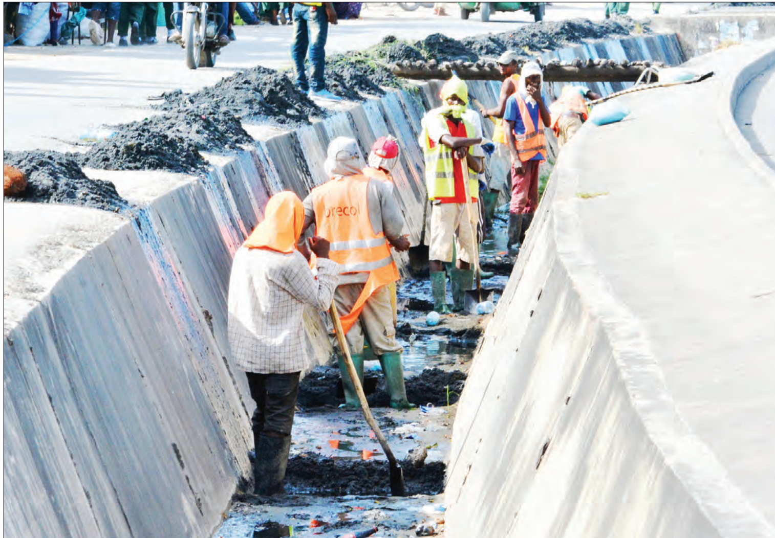
Youth volunteer to clear a clogged sewage system at River Side Ubungu in the outskirts of Dar es Salaam yesterday. Photo: Correspondent Miraji Msala
