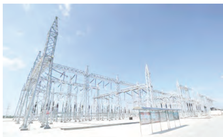
Photo shows the project where Myanmar's northern state of Kachin is connected with a 230KV backbone project.
