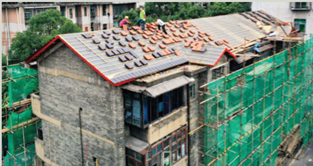
An old residential building in Shuangjiang township, Tongdao Dong autonomous county, Huaihua, central China's Hunan province is being renovated, Aug. 31, 2022. (Photo by Li Shangyin/People's Daily Online)
