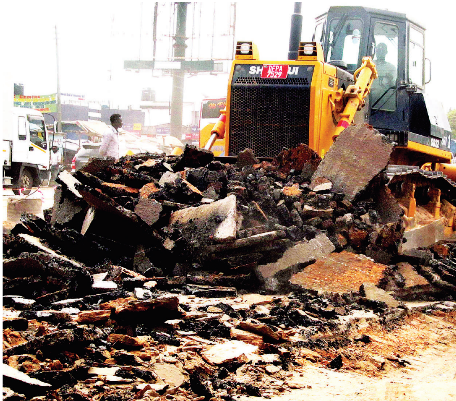
Implementation of Dar es Salaam's rapid transit road infrastructure project under way along the Mbagala Rangi-Tatu stretch of Kilwa Road yesterday. Photo: Correspondent Sabato Kasika
