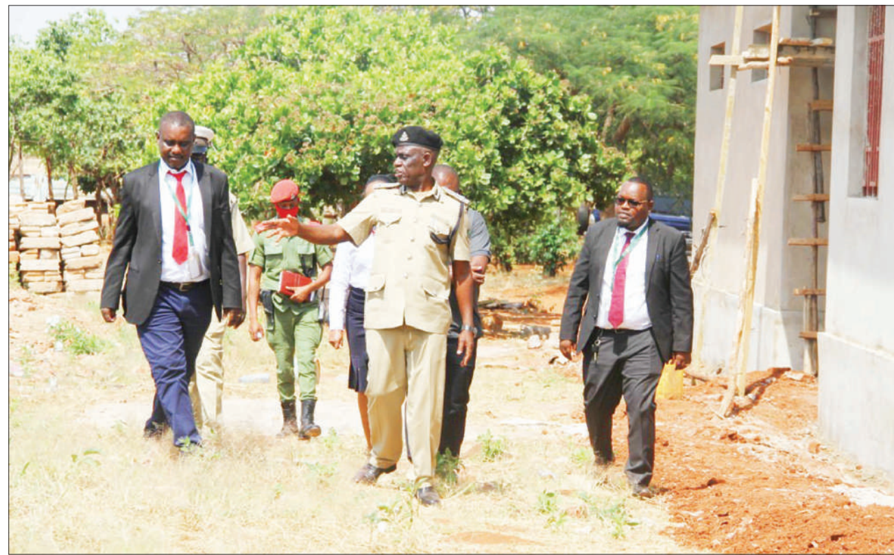
Dodoma Regional Police Commander Gilles Muroto leads TPB Bank Plc's Dodoma Branch manager, Shaban Telatela (L), at the weekend to the site where the construction of buildings for a police station at Mbande in Kongwa District is in progress. The bank has donated ten tonnes of cement worth 3m/- in support of the work. Photo: Guardian Correspondent
