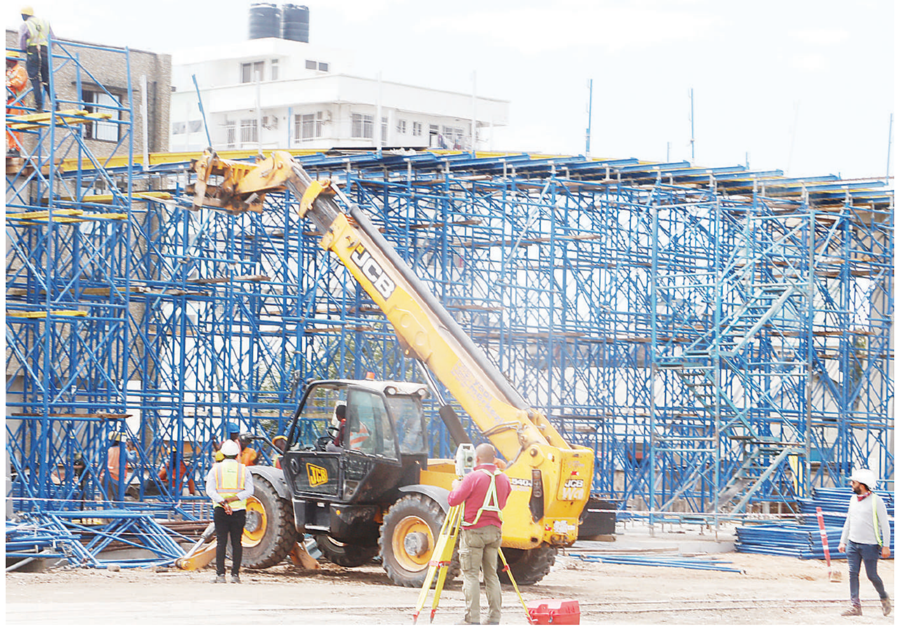
Work on Standard Gauge Railway infrastructure in progress under Yapi Markezi company contractors and technicians near Dar es Salaam's Karum Stadium yesterday. Photo: Correspondent Jumanne Juma
